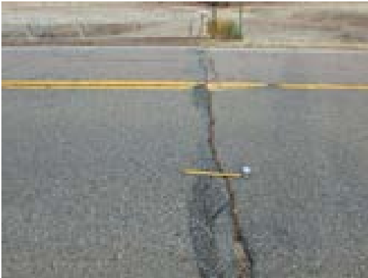
Figure 37: Bridge G-21-A – Major Cracking on the Bridge Deck Source: CDOT
