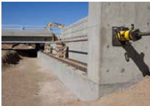
Figure 42: Use of Slide-In Method to Replace a Bridges Along State Highways 71 and 266
