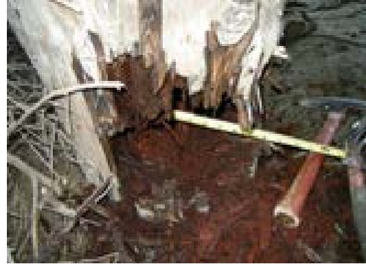
Figure 5: Bridge C-22-K – Rotted Supports
