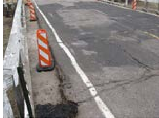
Photo 34: Bridge F-20-J – Deteriorating Bridge Deck Re-Asphalted Source: CDOT
