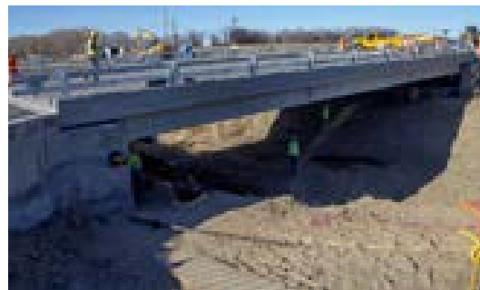
Figure 43: Use of Slide-In Method to Replace a Bridges Along State Highways 71 and 266
