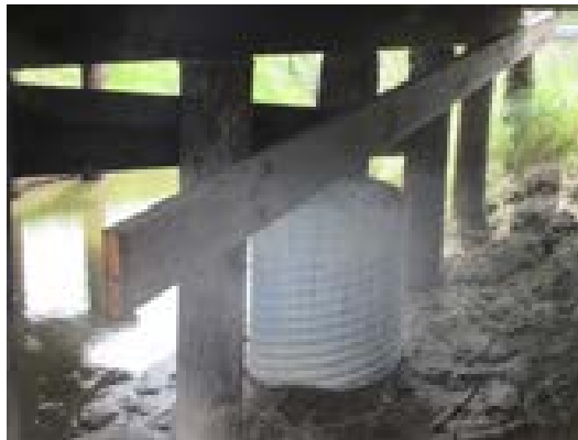
Figure 6: Bridge C-22-K – Concrete Collars to Address Rotted Supports
