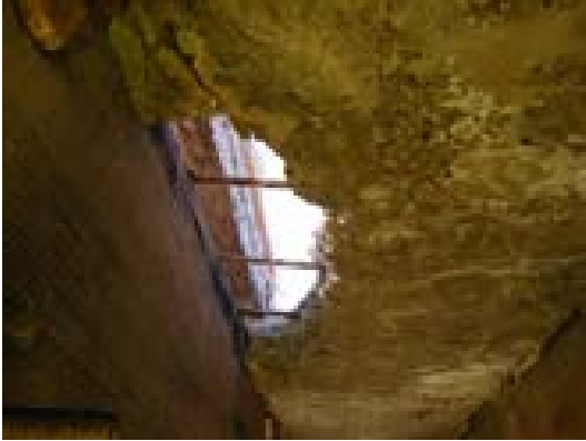
Figure 33: Bridge F-20-J – Hole on the Edge of the Bridge Deck Source: CDOT
