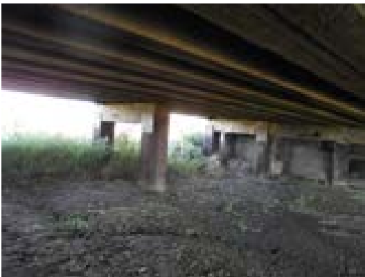
Figure 23: Bridge F-19-E – Wooden Bents Supporting Stringers to Maintain Structural Integrity of the Superstructure Source: CDOT
