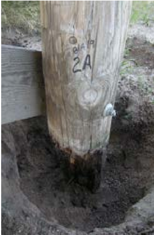
Figure 14: Bridge D-25-E – Rotting Timber Support Source: CDOT
