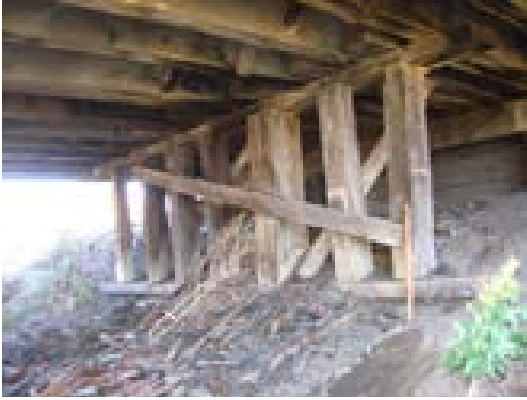
Figure 4: Bridge C-22-K – Wooden Bents to Maintain Structural Integrity of the Superstructure
