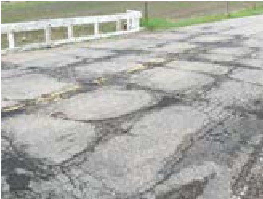
Figure 28: Bridge F-20-L – Condition of Bridge Deck Source: CDOT
