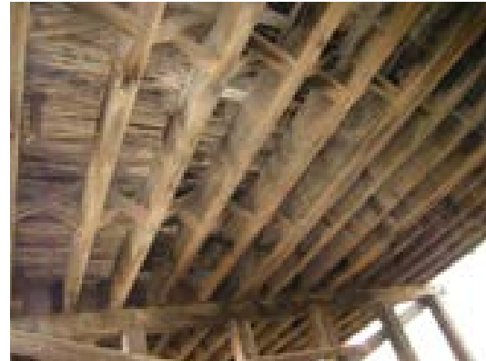
Figure 38: Bridge G-21-A – Damp and Rotting Stringers Under the Span Source: CDOT
