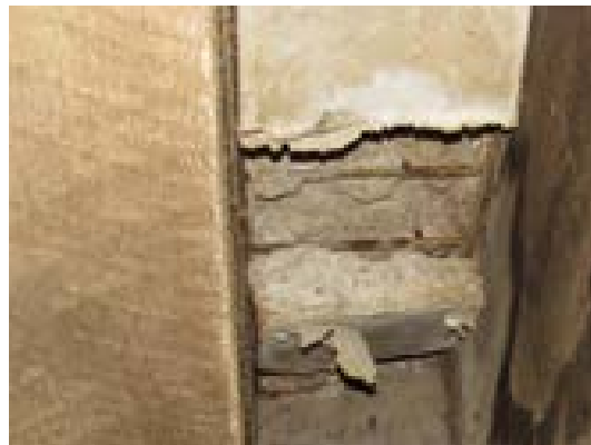
Figure 24: Bridge F-19-E – Missing Concrete and Exposed Rebar Source: CDOT
