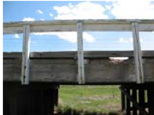
Figure 29: Bridge F-20-L – Rotted Posts, Rusted-Out Anchor Bolts and Deteriorating Deck Source: CDOT
