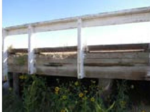
Figure 25: Bridge F-19-E – Rotten Wooden Stringer and Deterioration of Deck Source: CDOT
