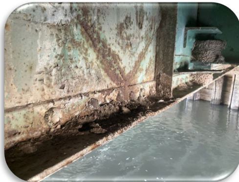
Corrosion along riveted girder bottom flange at J-04-X
