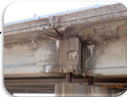
Deteriorated girder end at C-22-BG
