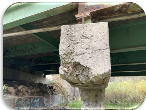
Pier cap spalling on P-05-B
