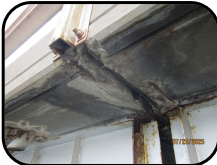
Overhang Deterioration at Joint Location
