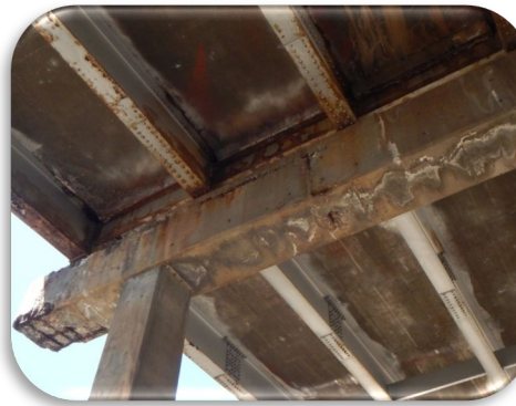
Spalling and exposed corroded rebar of pier
