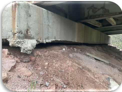
Active washing below abutment
