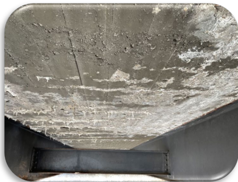
Heavy efflorescence in bay at midspan
