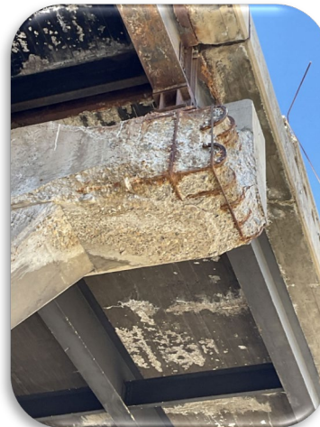
Pier with exposed, corroded rebar
