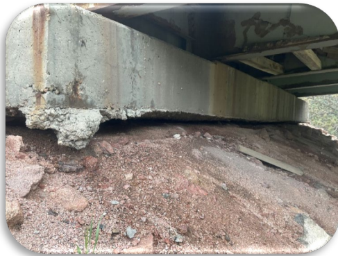
Active washing below abutment
