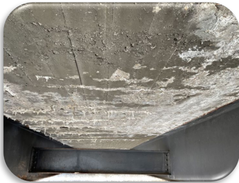
Heavy efflorescence in bay at midspan
