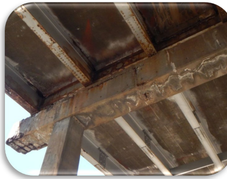
Spalling and exposed corroded rebar of pier
