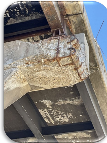
Pier with exposed, corroded rebar
