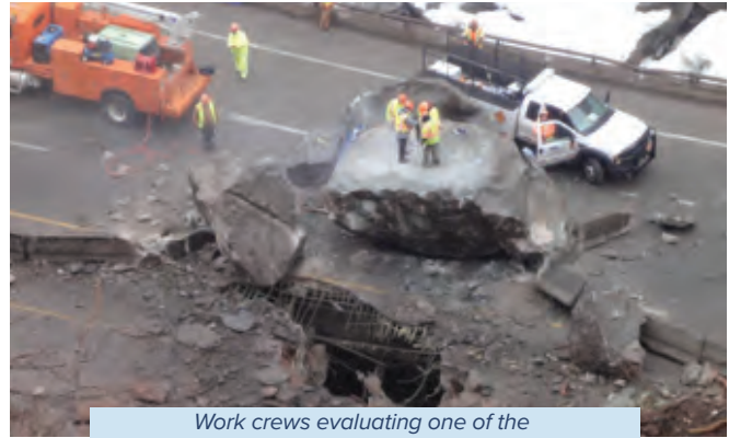
Work crews evaluating one of the large boulders from the 2010 incident.
