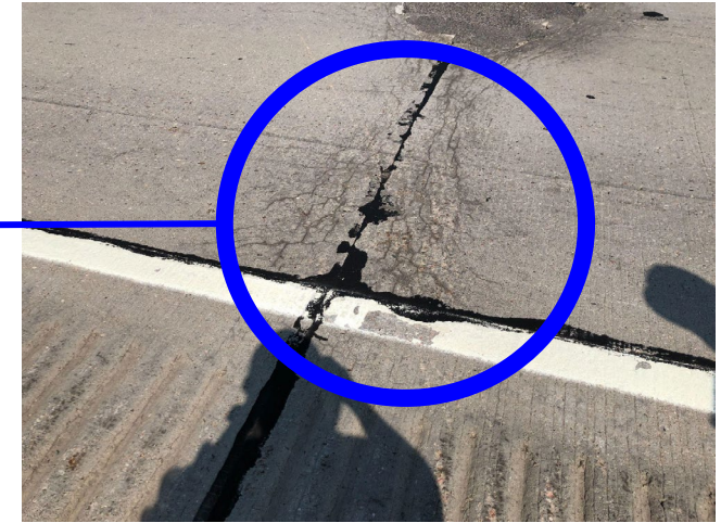
Alkali-silica reactivity (ASR) distress
