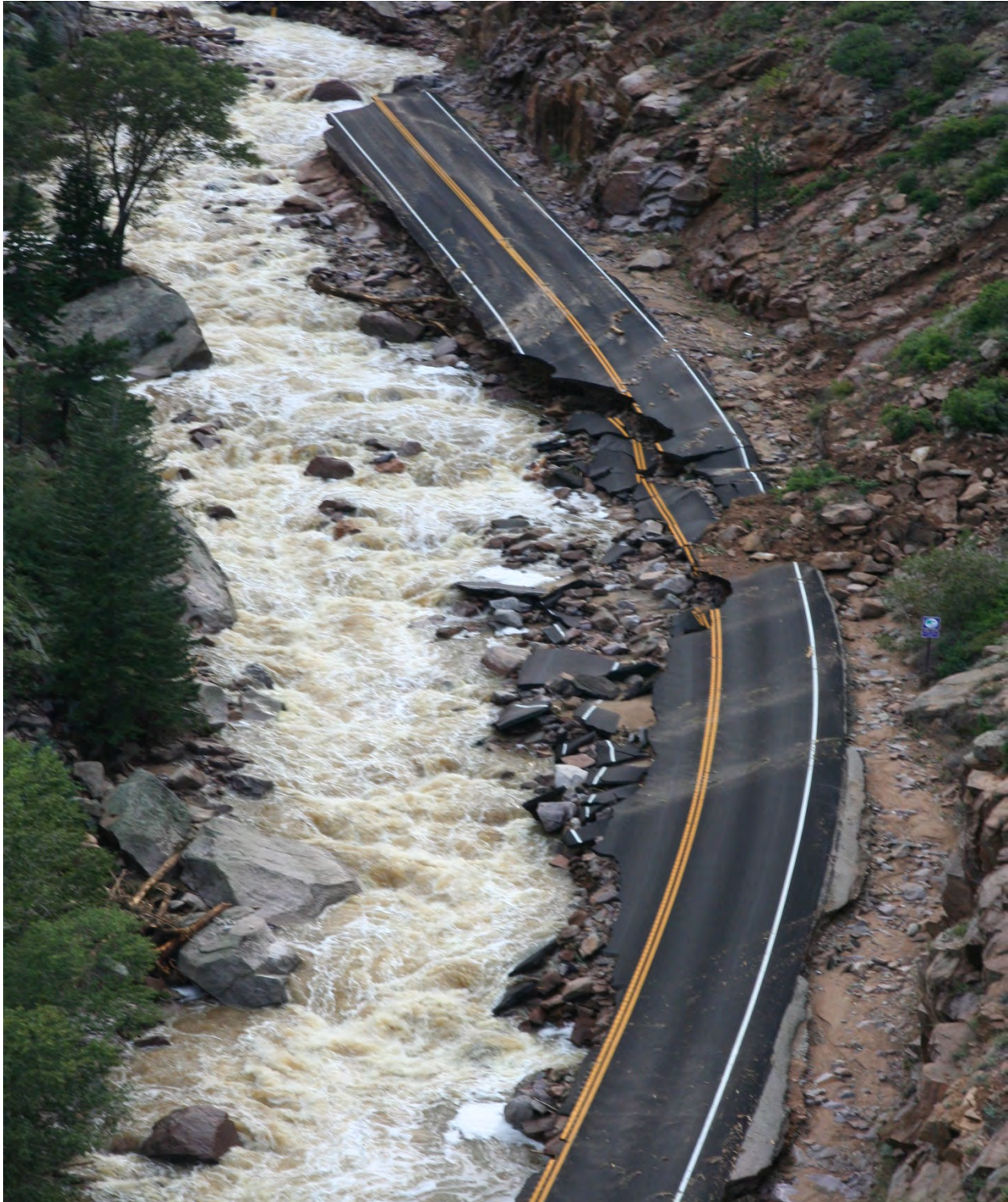
Figure 36 - MP 26.9, Roadway undermined and washed out embankment.
