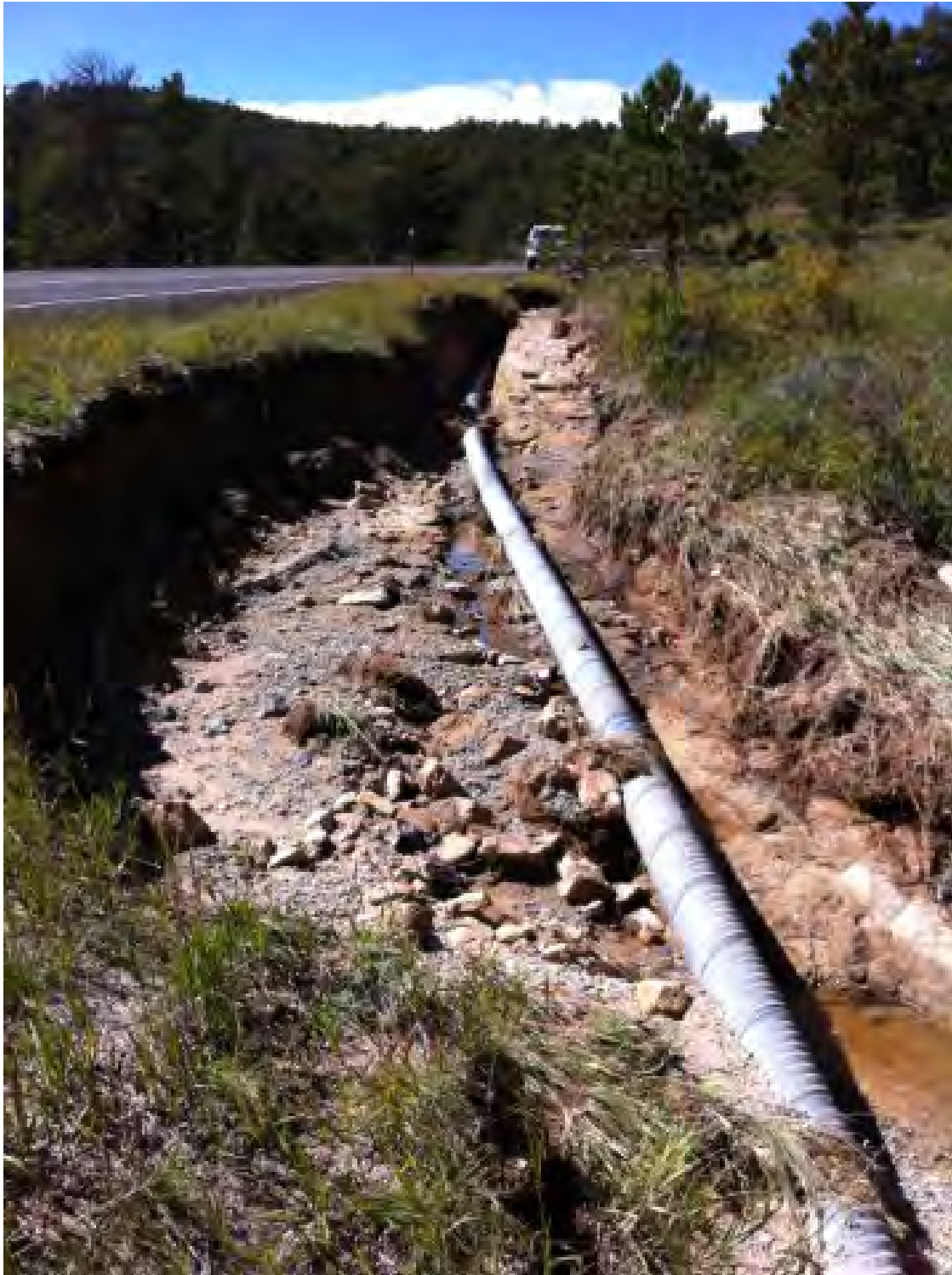
Figure 9 - MP 19.15, Eastbound ditch damage.
