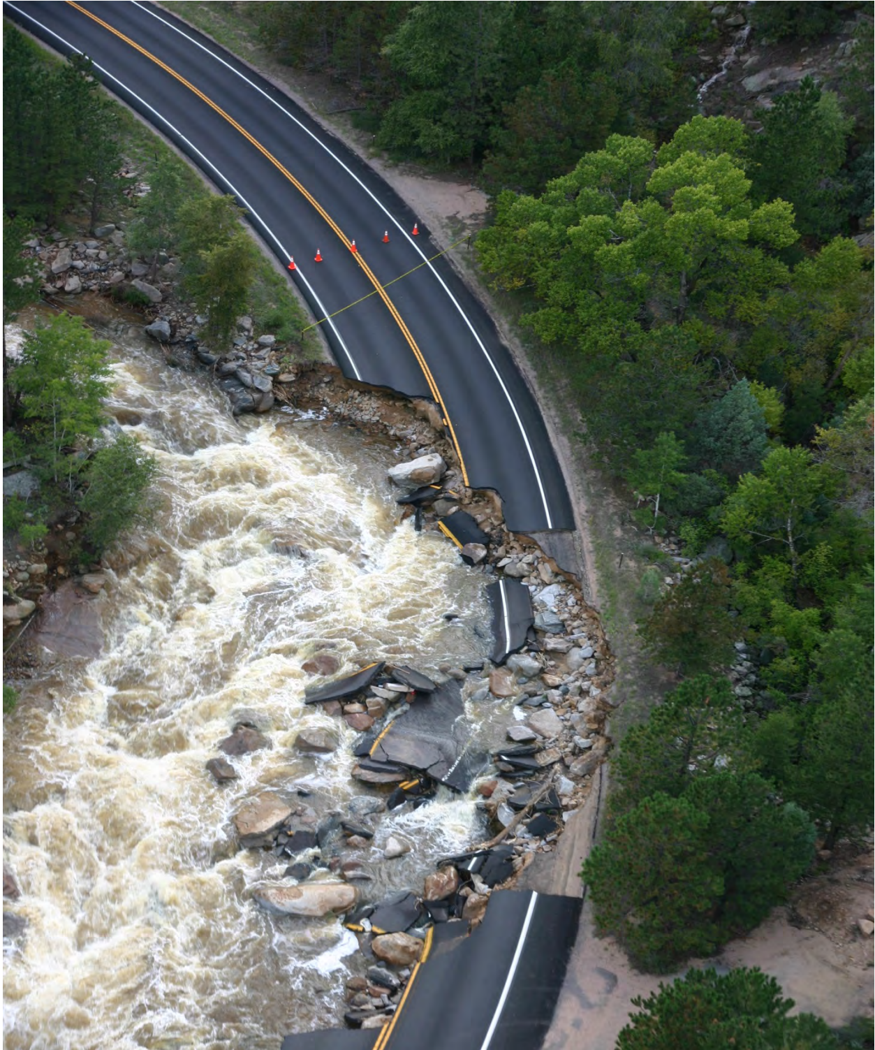
Figure 25 - MP 23.8, Complete 2 lane roadway wash out.
