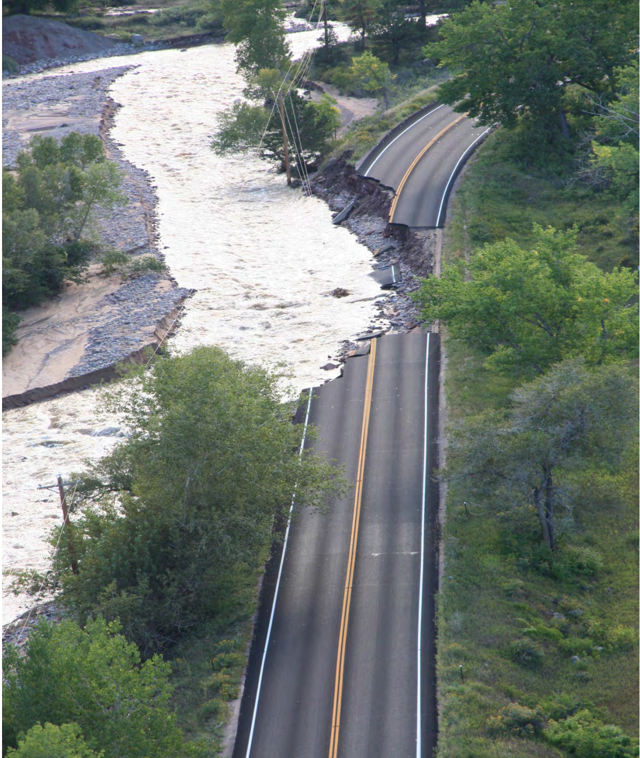
Figure 44 - MP 30.49, Complete roadway loss
