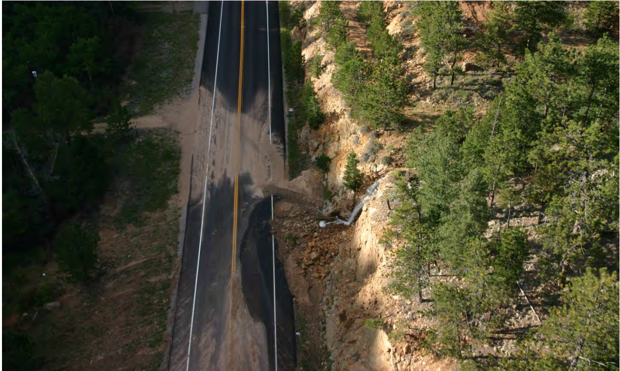
Figure 13 - MP 21.68, Material slide onto road.
