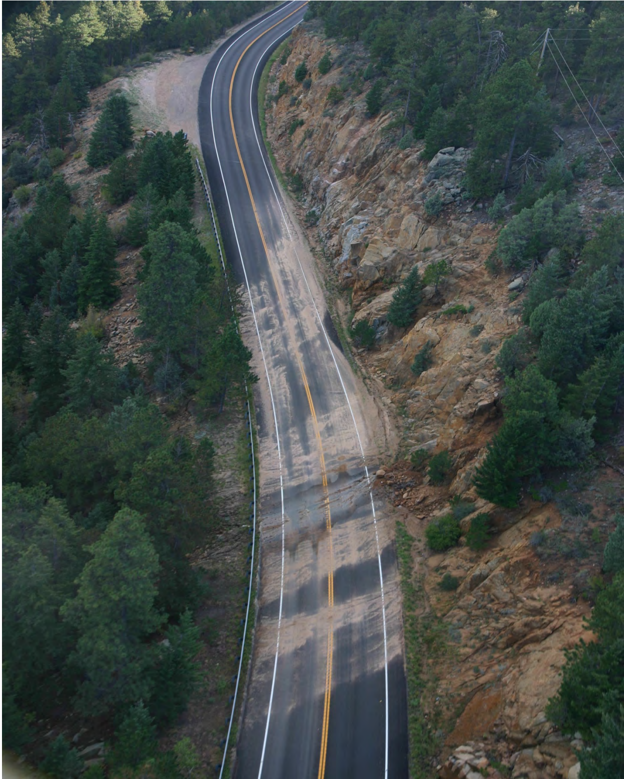
Figure 12 - MP 20.86, Material slide onto road.
