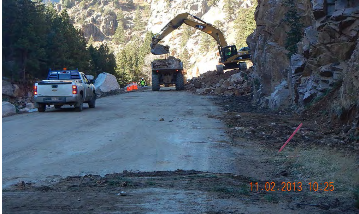
Figure 53 - MP 26.2 Facing west, Clearing rockfall.
