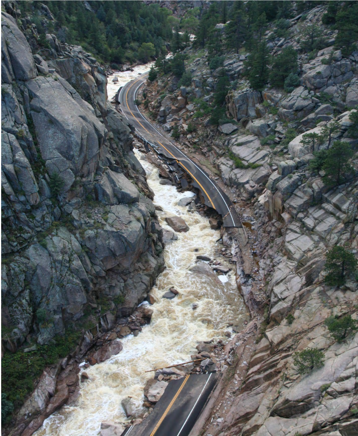
Figure 39 - MP 27.68, Wash out of riverside embankment and roadway due to lateral scour and overtopping of the roadway.
