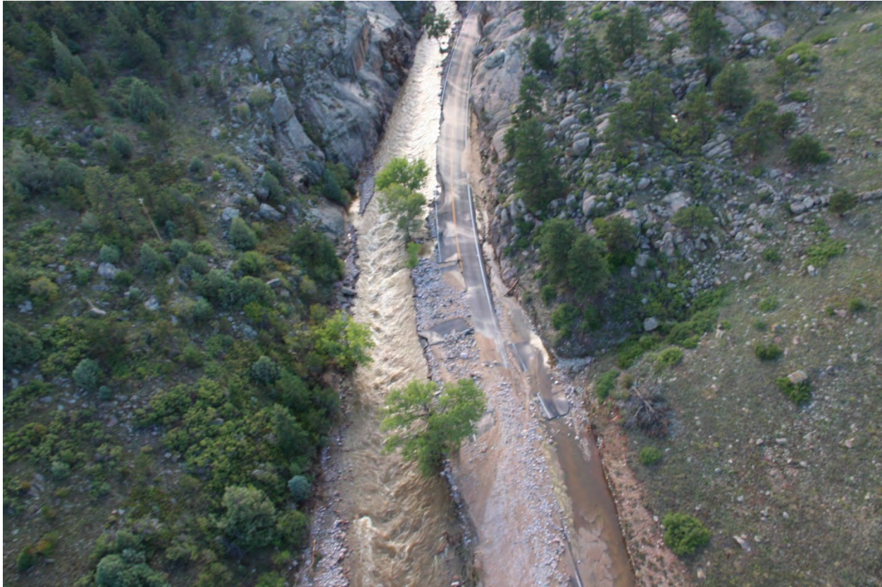
Figure 42 - MP 30.08, Wash out of the roadway embankment and pavement due to lateral scour and overtopping of the roadway. Sediment and debris deposition throughout.
