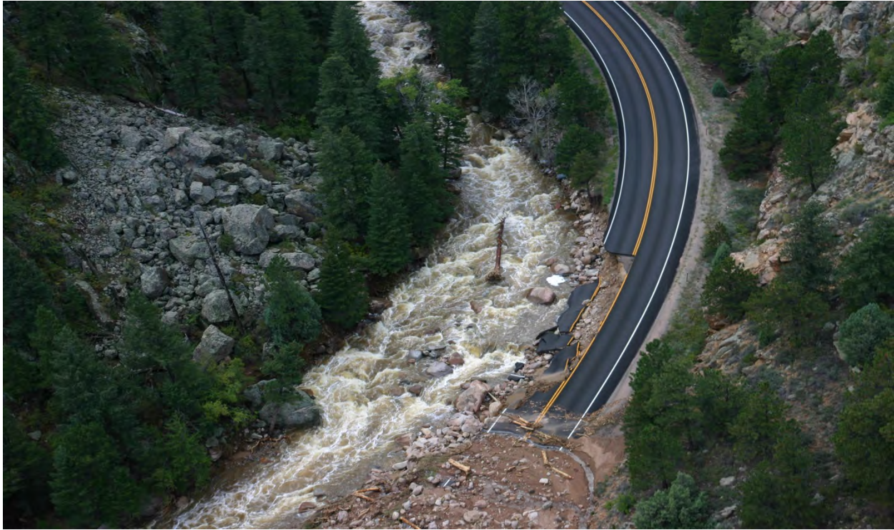
Figure 28 - MP 24.75, Rock slide and debris covering roadway lanes, embankment and roadway washout.
