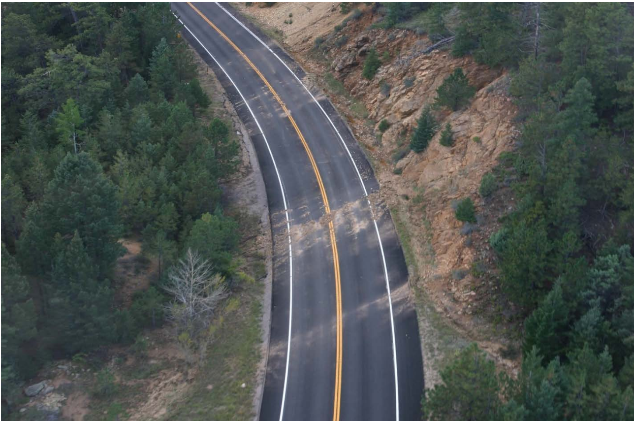
Figure 11 - MP 20.66, Westbound ditch damage and material slide.
