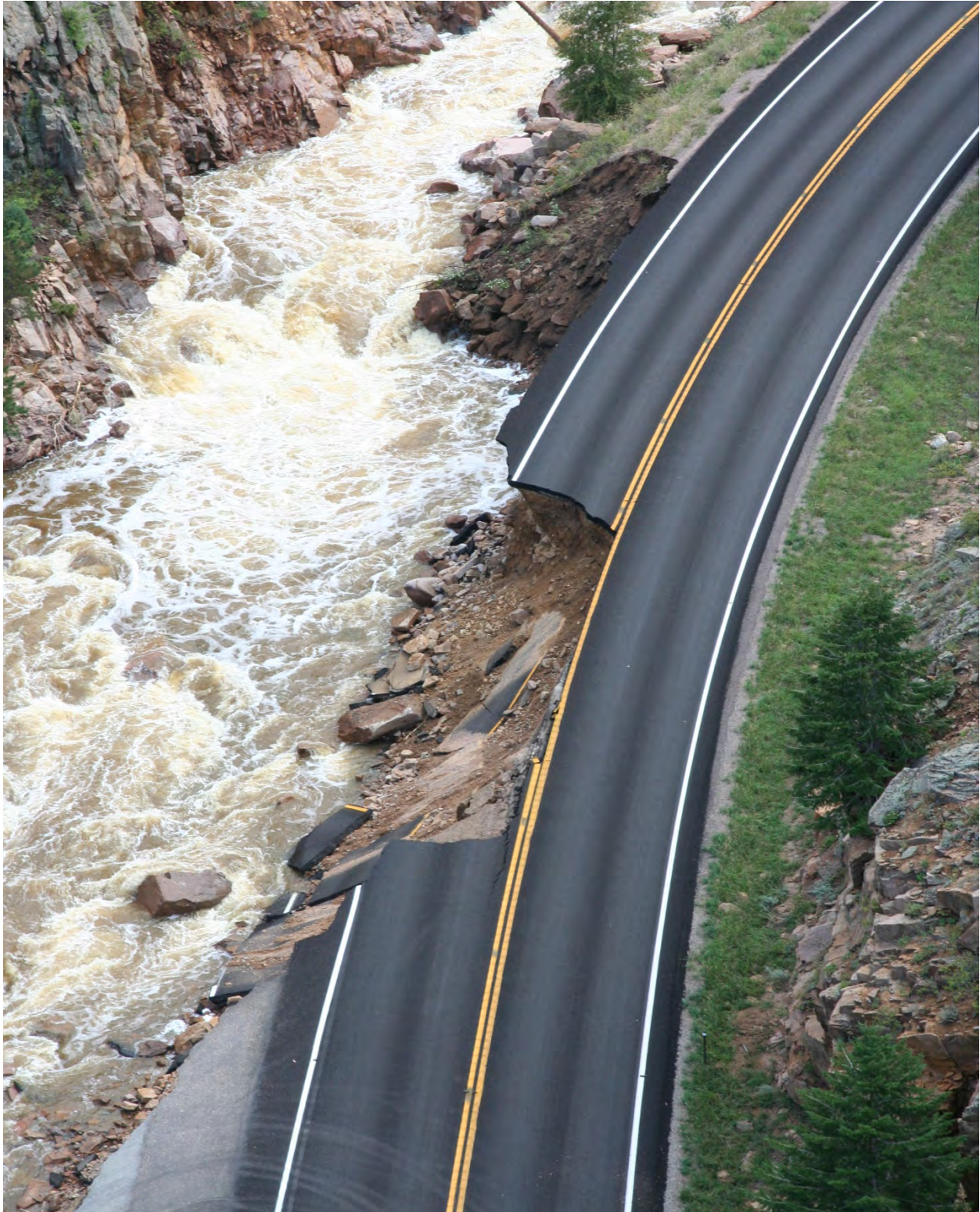
Figure 31 - MP 25.75, Embankment and partial roadway washout.
