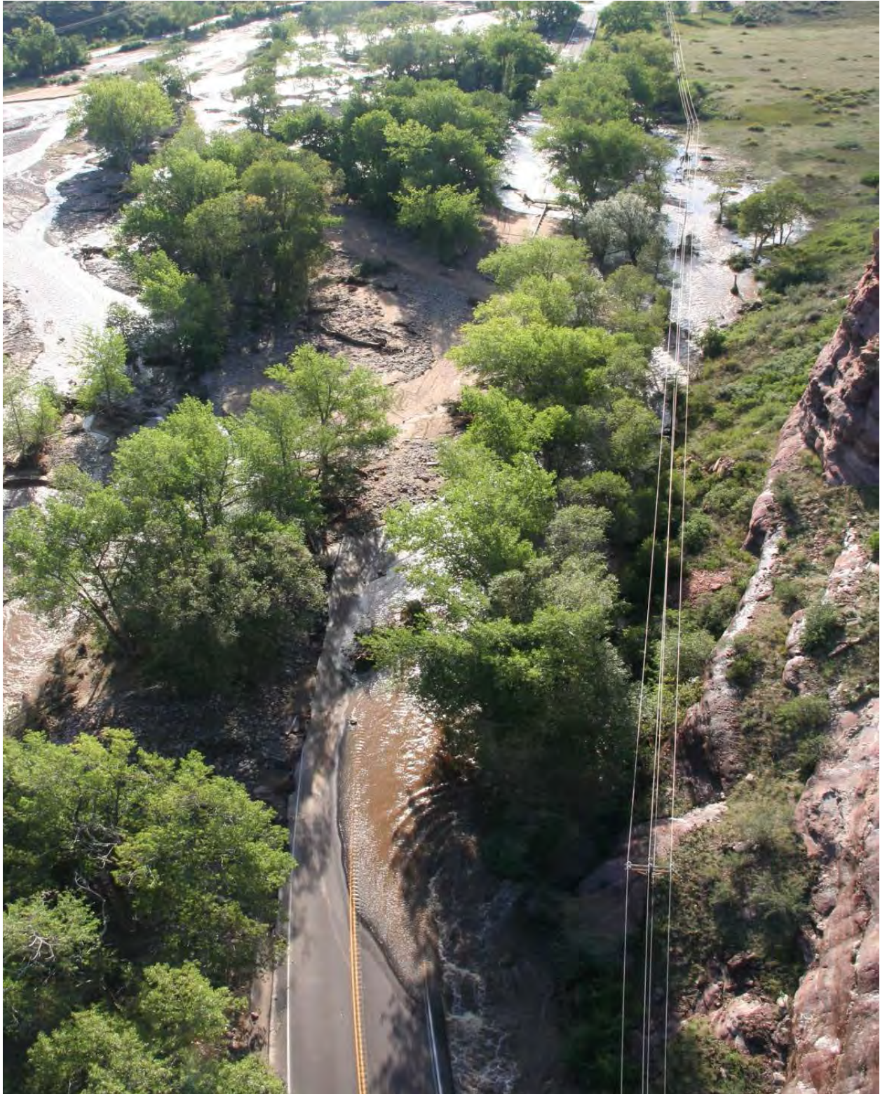
Figure 65 - MP 31.64, Roadway overtopped throughout section, shoulder and ditch washouts on both sides.
