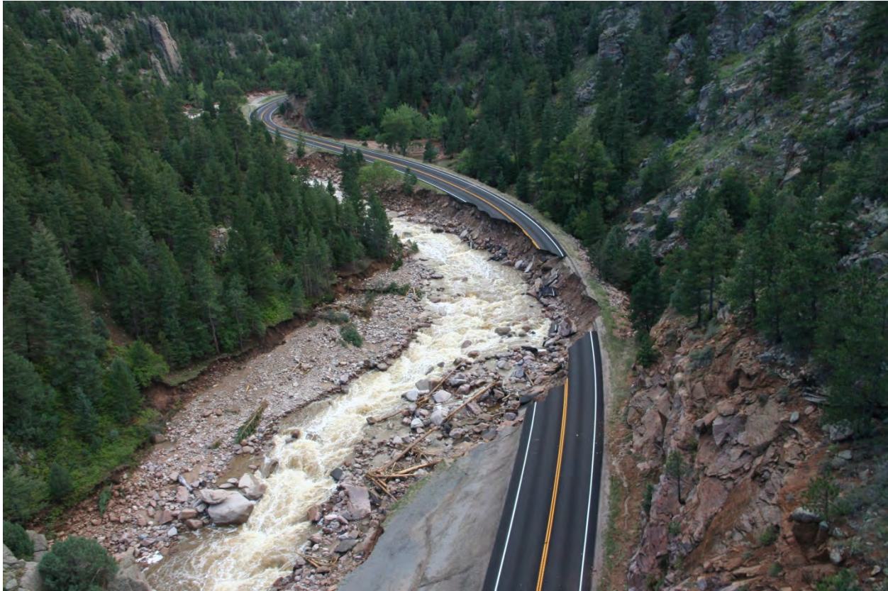
Figure 37 - MP 27.28, Complete roadway loss due to embankment scour damage at the river bend.
