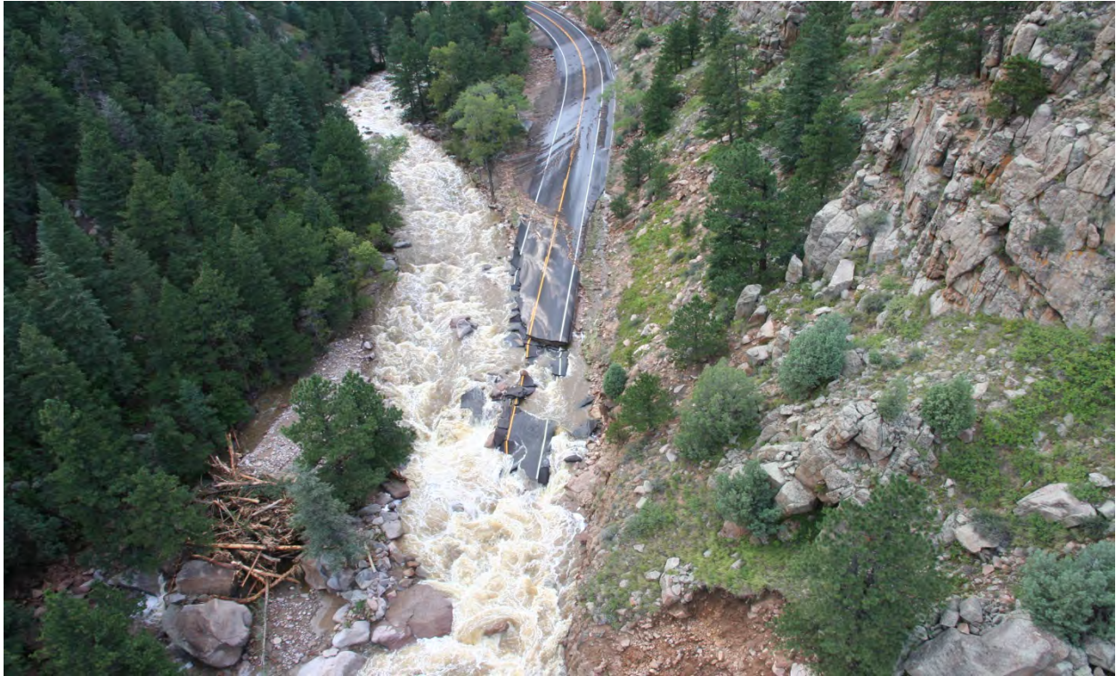
Figure 34 - MP 26.61, Complete roadway loss due to overtopping.
