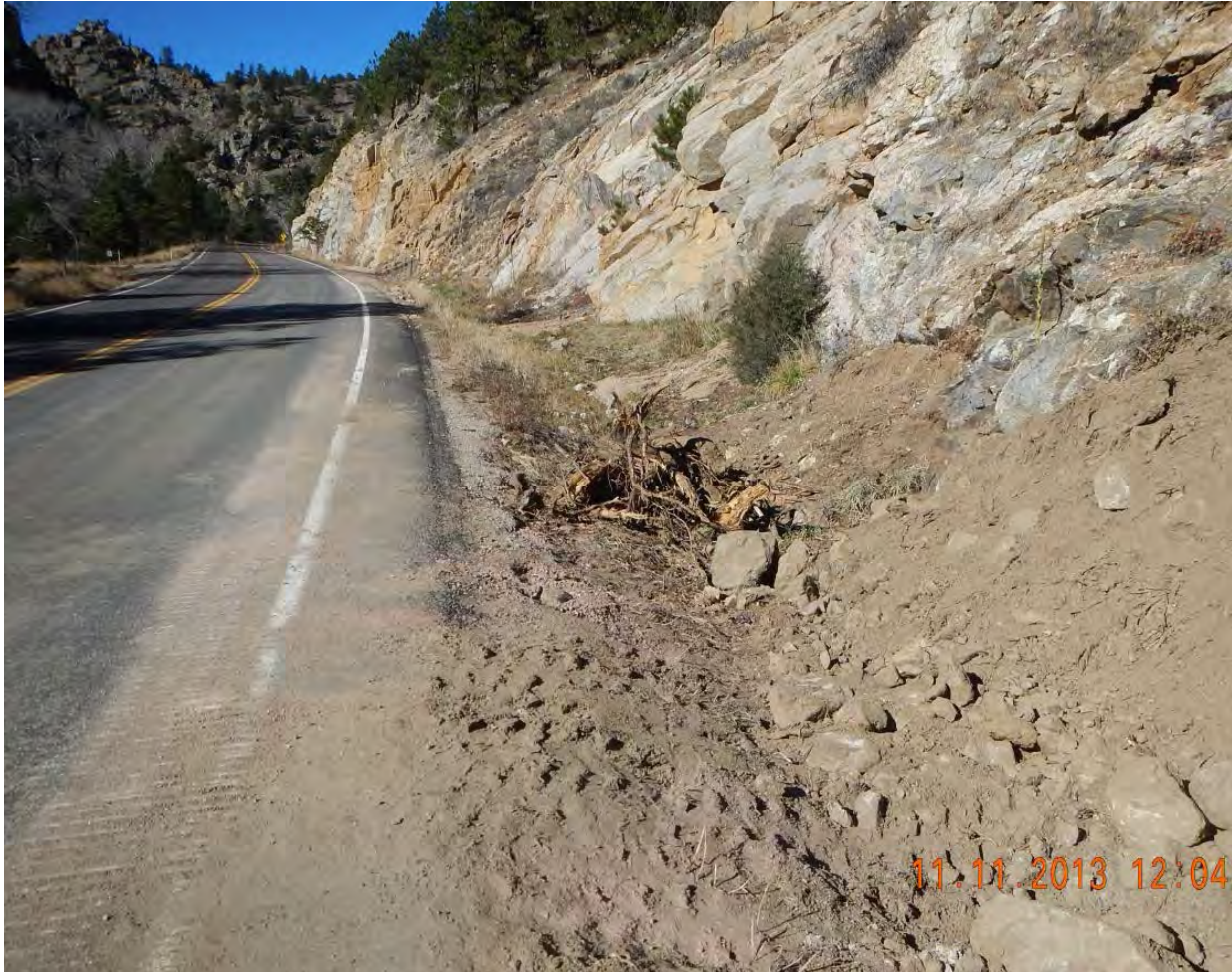
Figure 21 - MP 22.95, Removal of material from slide and regarding of westbound roadside ditch.
