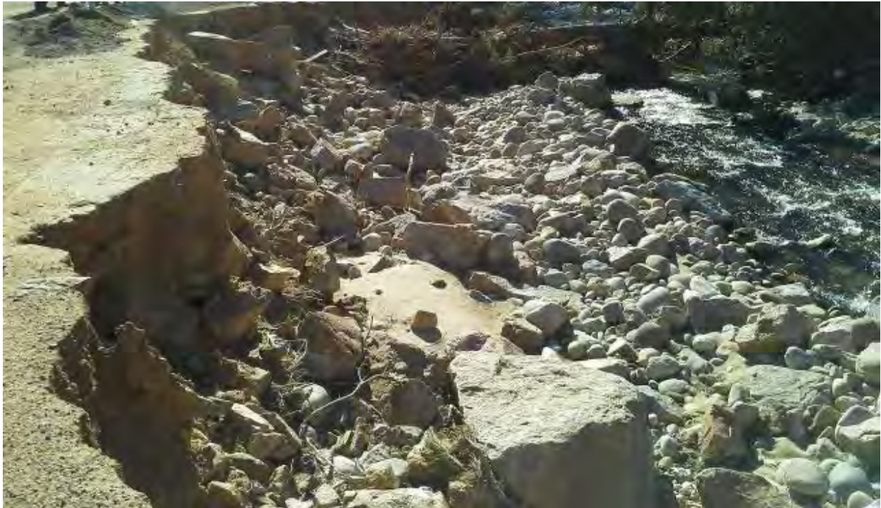
Figure 17 - MP 22.13, Eastbound roadway embankment scour damage.
