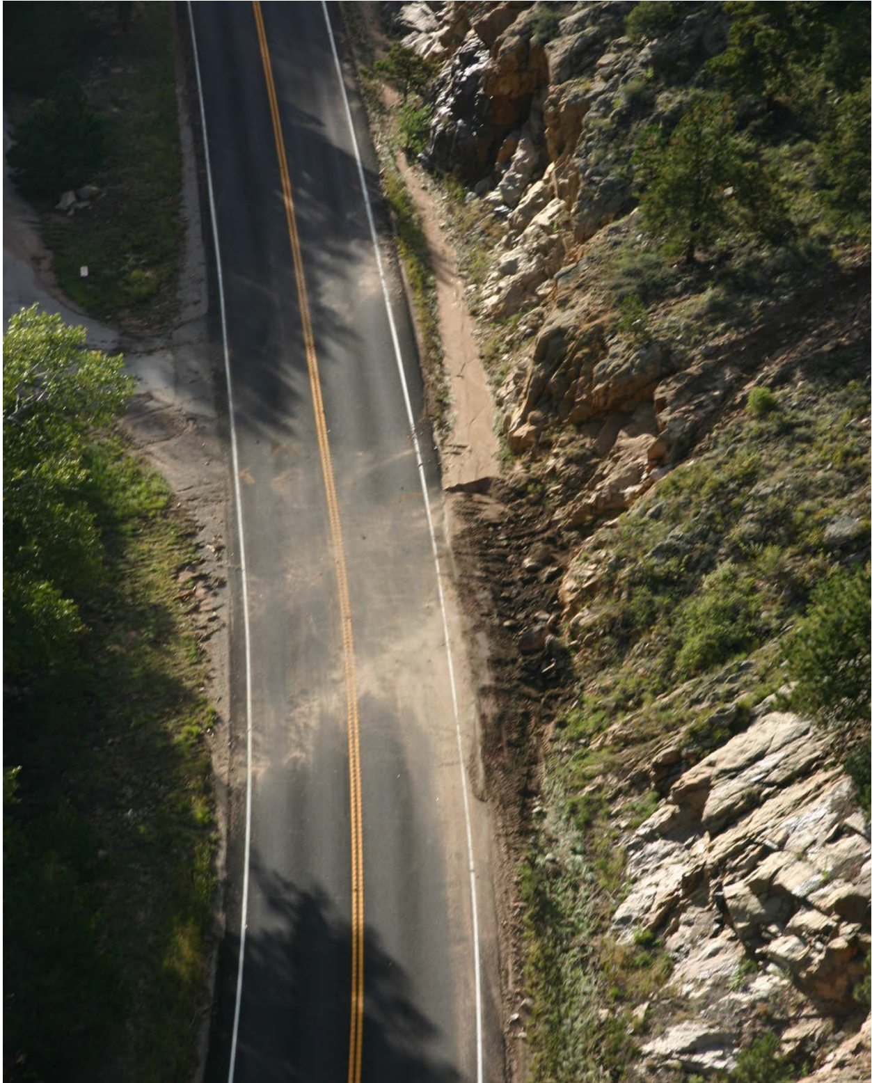
Figure 19 - MP 22.83, Material slide onto roadway.
