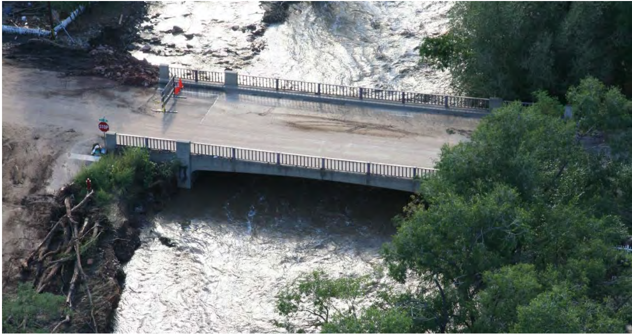
Figure 76 - MP 32.98, Structure D-15-A with abutment scour and undermined pavement behind abutment.
