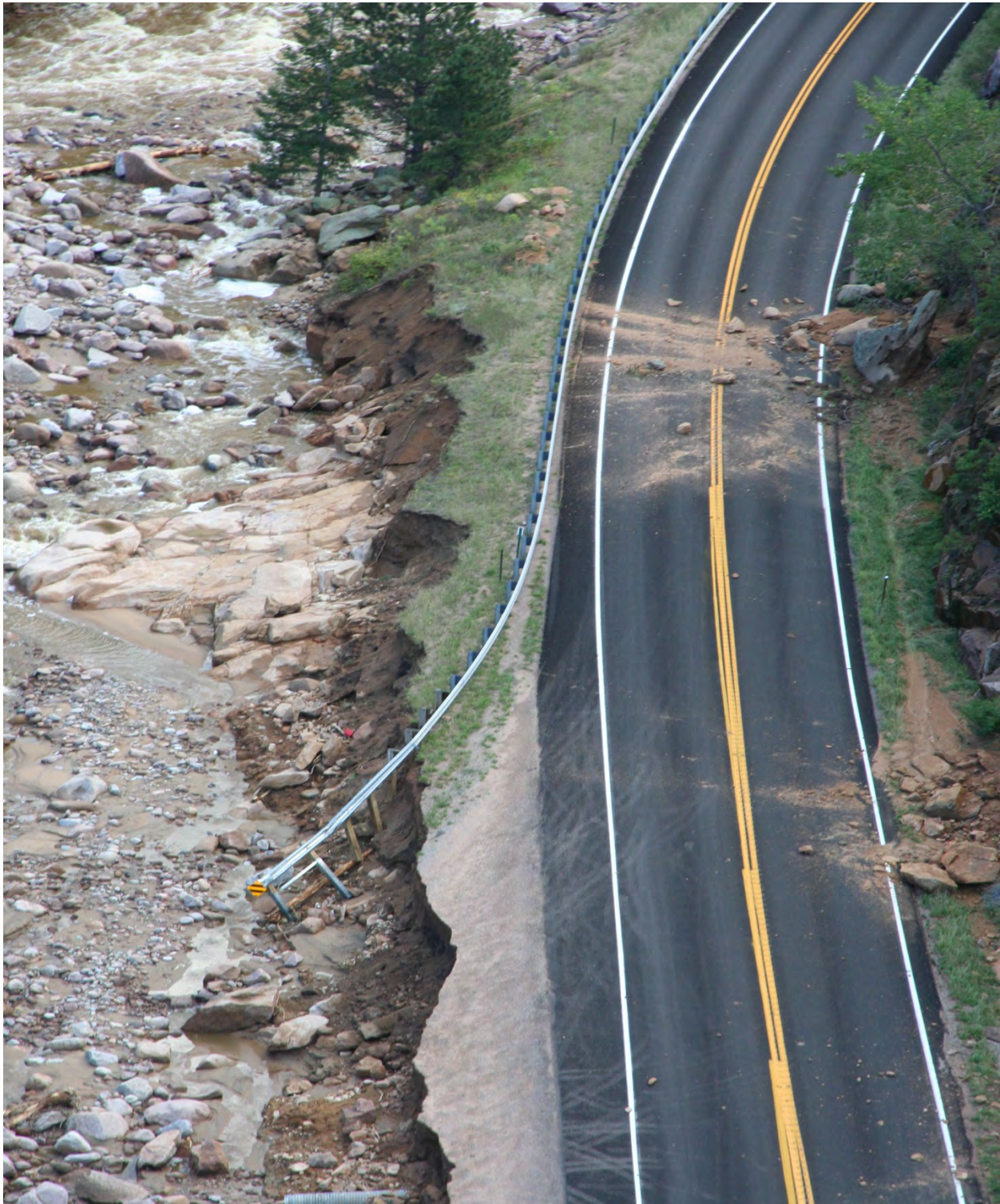
Figure 40 - MP 28.3, Scour damage to gravel pullout, EB embankment and guardrail; and material slides.
