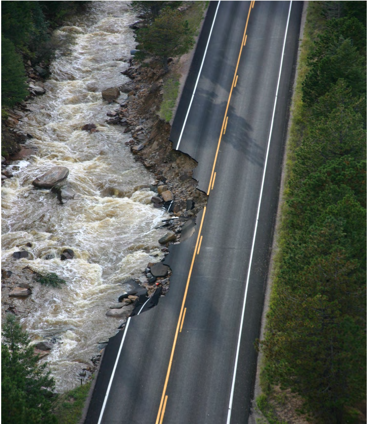
Figure 24 - MP 23.54, Roadway embankment damage, partial wash out of EB lane.
