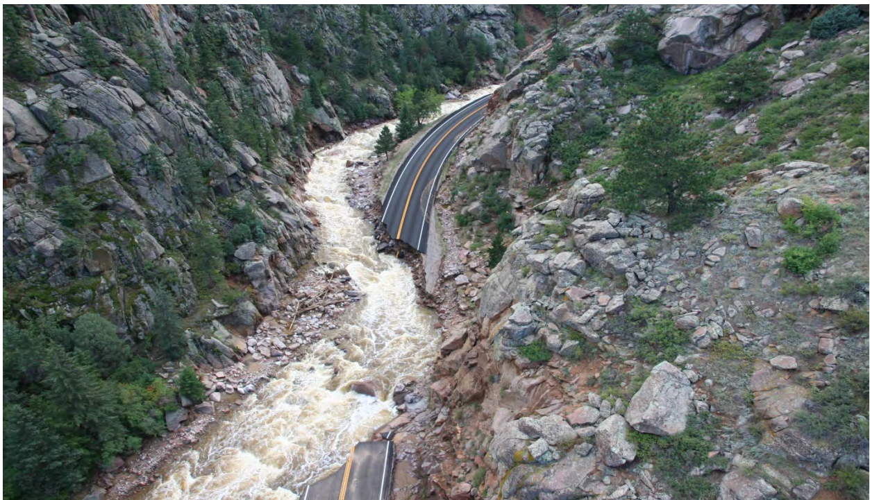
Figure 35 - MP 26.9, Complete roadway loss due to overtopping at the river bend
