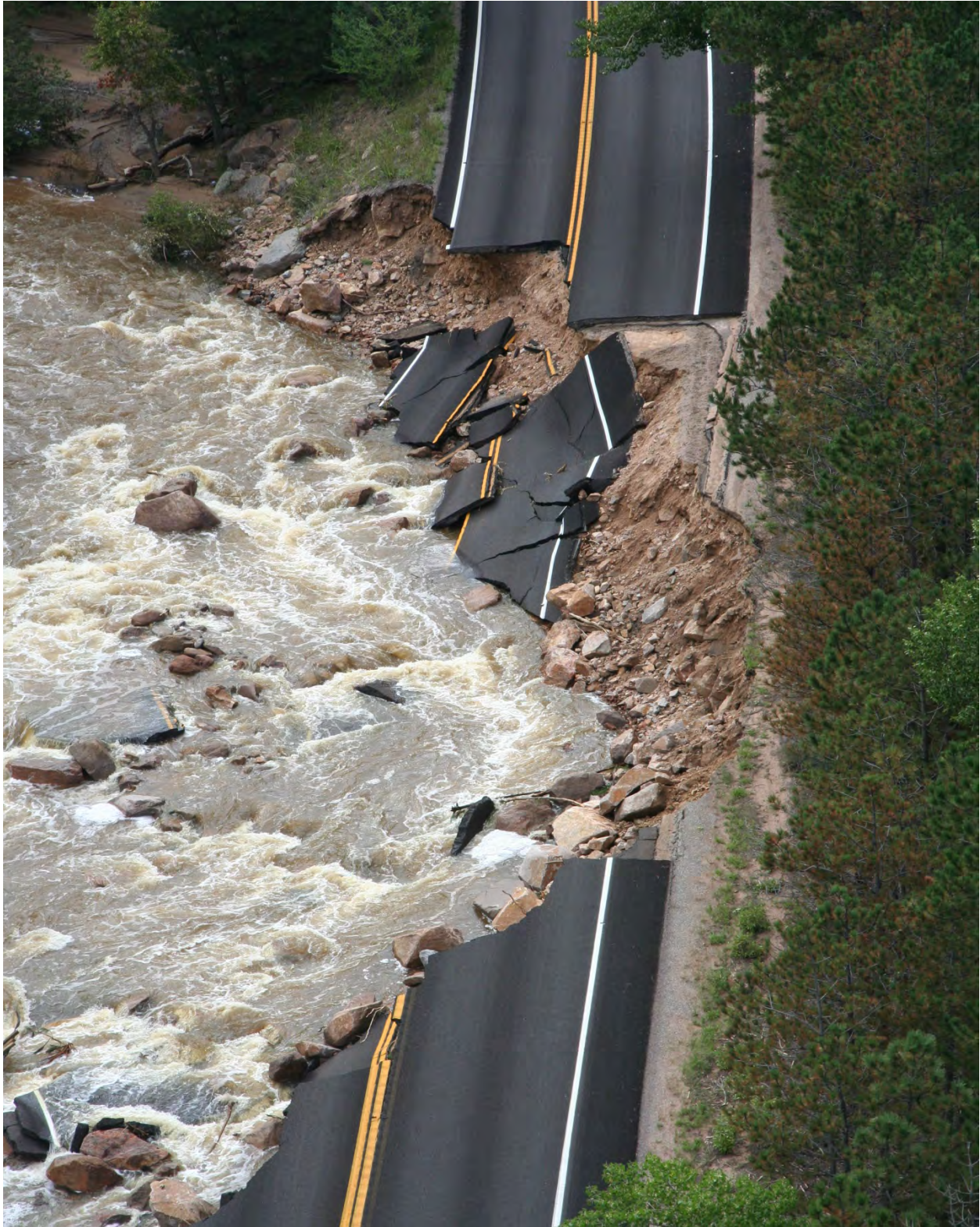
Figure 30 - MP 25.5, Embankment and roadway washout.
