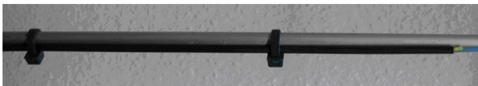
Figure 48: Sensor cable mounted with cable ties
