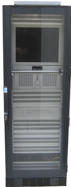
Figure 14: 19-inch rack comprising controller, computer and UPS
