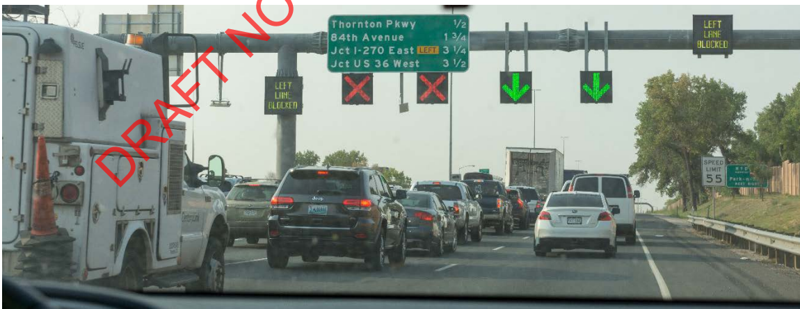
Figure 26 - Southbound I-25 queue warning system 0.5 miles north of Thornton Pkwy
