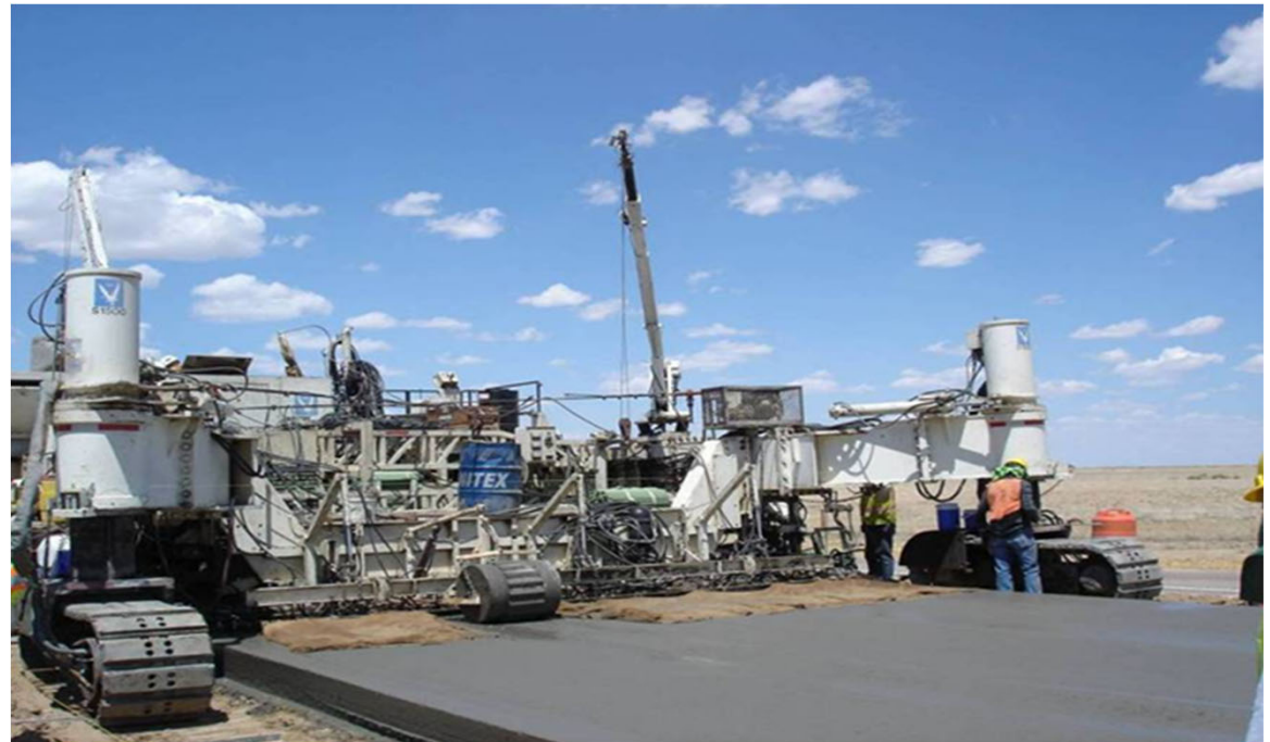
1 st CDOT Paving Project w/ PLC US 287 (Ports to Plains route) in eastern CO
