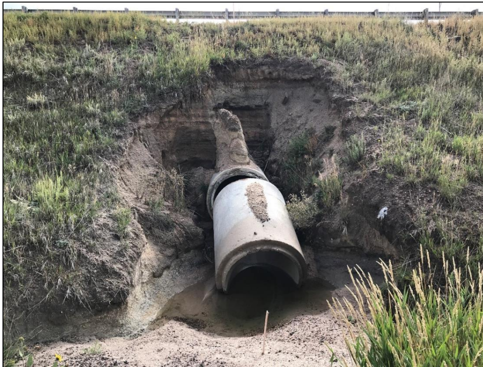
Photo 11.1 Culvert outlet failure on I 25 near milepoint 162.1, 9/6/2018
