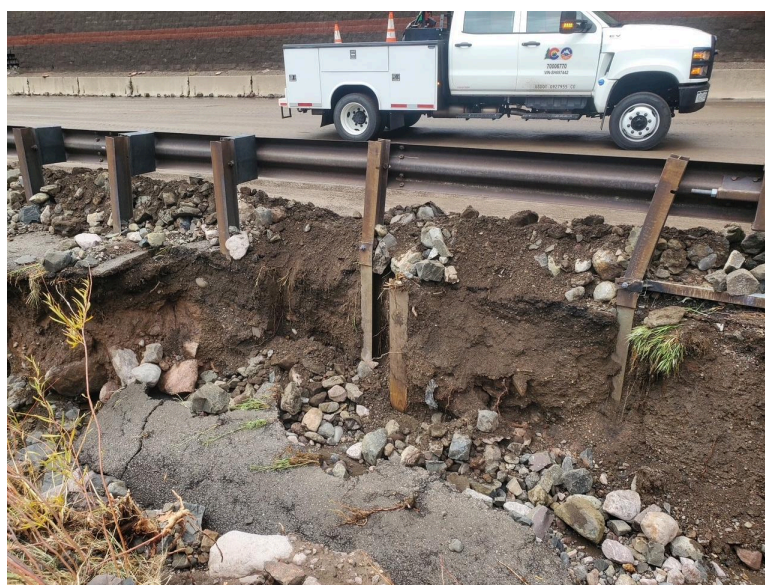
Retaining wall damage on US 160 at MP 161
