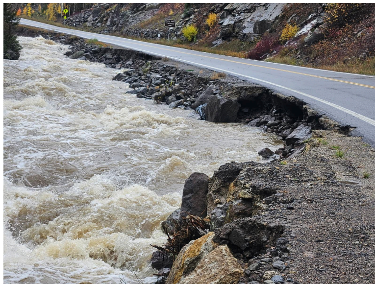
Shoulder damage and undercutting of the roadway on US 160 at MP 177
