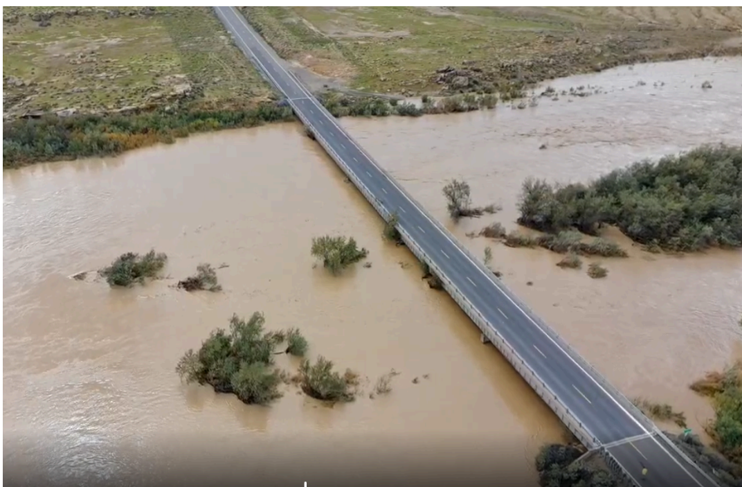
San Juan River Bridge and floodwaters reaching the bridge girders on US 160 at MP 1
