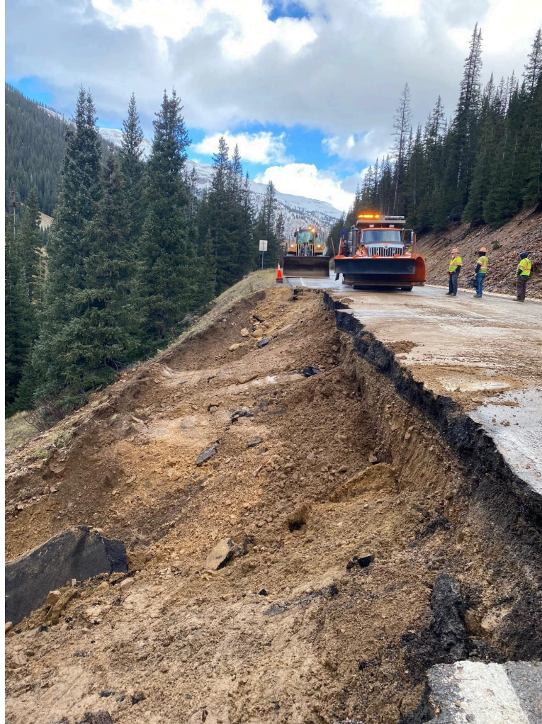
Damage to shoulder and southbound travel lane on US 550 at MP 75
