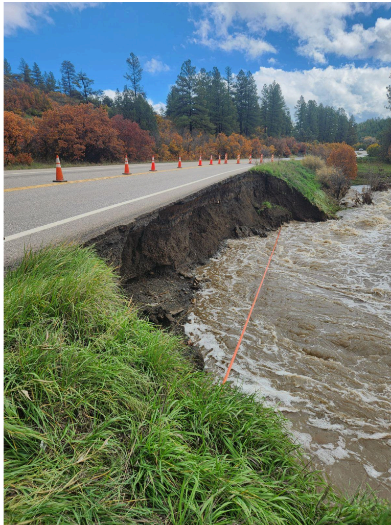
Significant shoulder damage and undercutting of travel lanes on US 160 at MP 135
