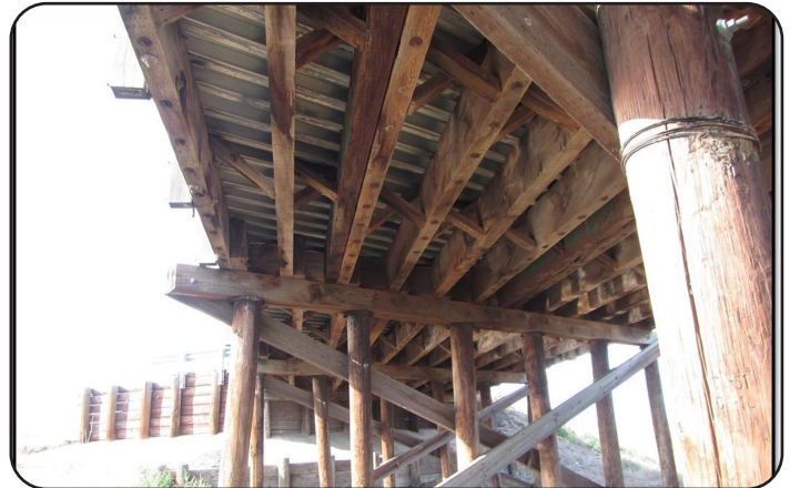
Image 6. Existing Split Timber Stringer Repair on US 36 over Vega Creek in Washington County (F-22-V)
