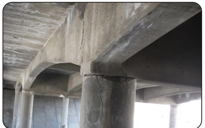
Image 8. Girder and Pier Column Cracks on I-70 ML over Harlan St in Jefferson County (E-16-FZ)
