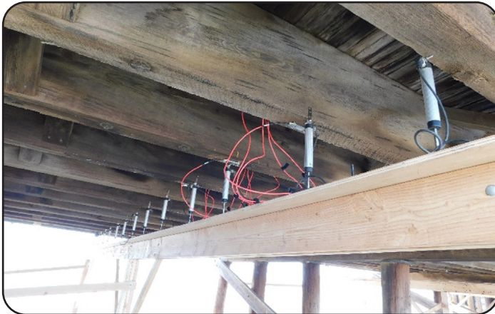
Image 5. Load Testing Sensors Measuring Displacement on US 36 over Vega Creek in Washington County (F-22-V)
