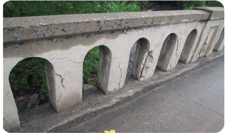
Image 12. Cracks in SH 7 WBND over Boulder Creek Bridge Rail (D-15-AQ)
