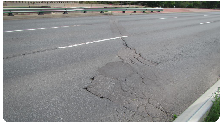
Image 14. Cracks and Potholing in SH 7 EBND over Boulder Creek Deck (D-15-AV)
