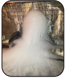
Image 16. Ice Build-up on the EJMT Liner
