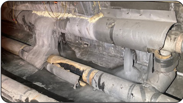
Image 16. Ice Buildup on the EJMT Plenum Liner
