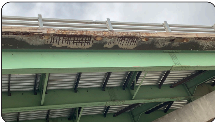
Image 6. Exposed Rebar and Deterioration to Deck Underside on I-270 WBND over Service Road, BNSF, RR
