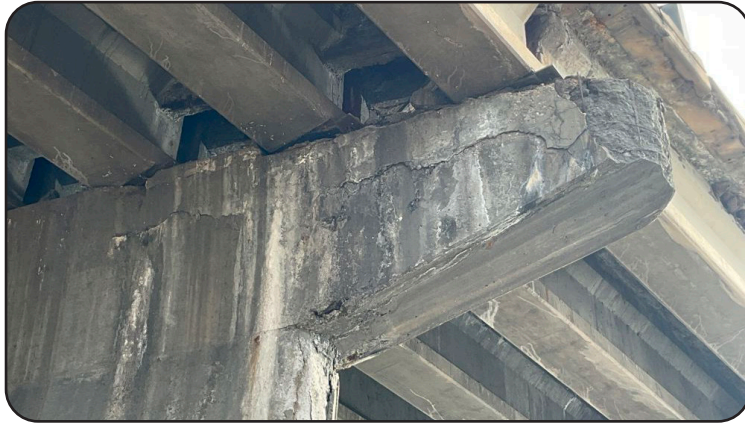
Image 4. Spalling and Deterioration to Superstructure on I-270 EBND over South Platte River
