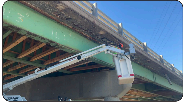
Image 5. Repairs to the Deck Underside on I-270 WBND over Ditch Road, Burlington Canal
