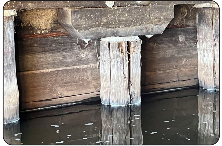
Image 9. Cracks in Timber Pile of US 40 ML over Shelton Ditch
