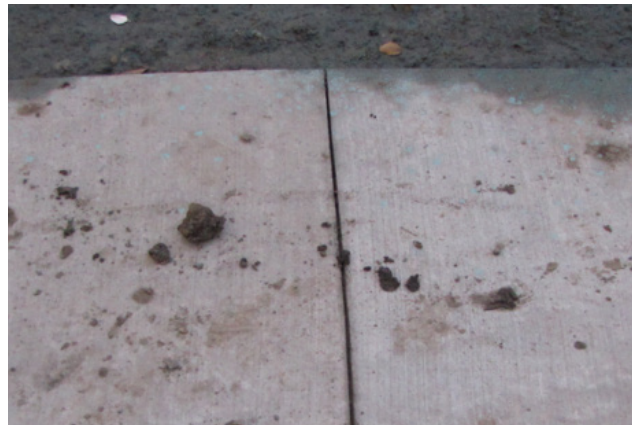
Saw cut joints offer a smoother ride for bicyclists
