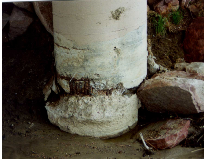
Fig. 16.12(D)-5 Photo of Damage to be repair by (D)-4 details
