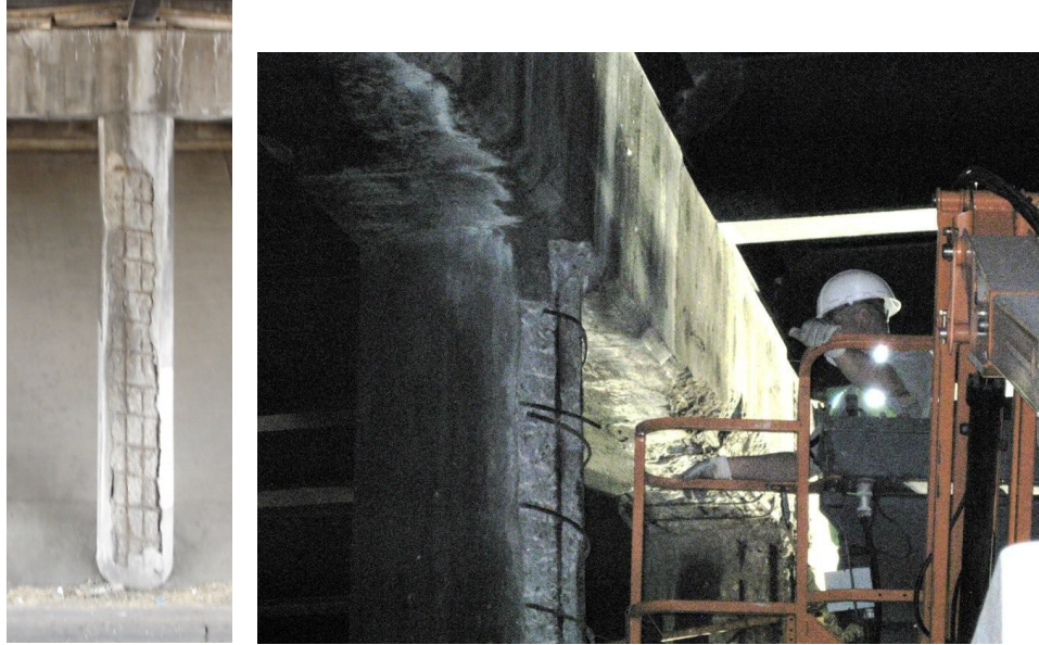
Fig. 16.12(D)-3 Photos showing column damage and repair process
