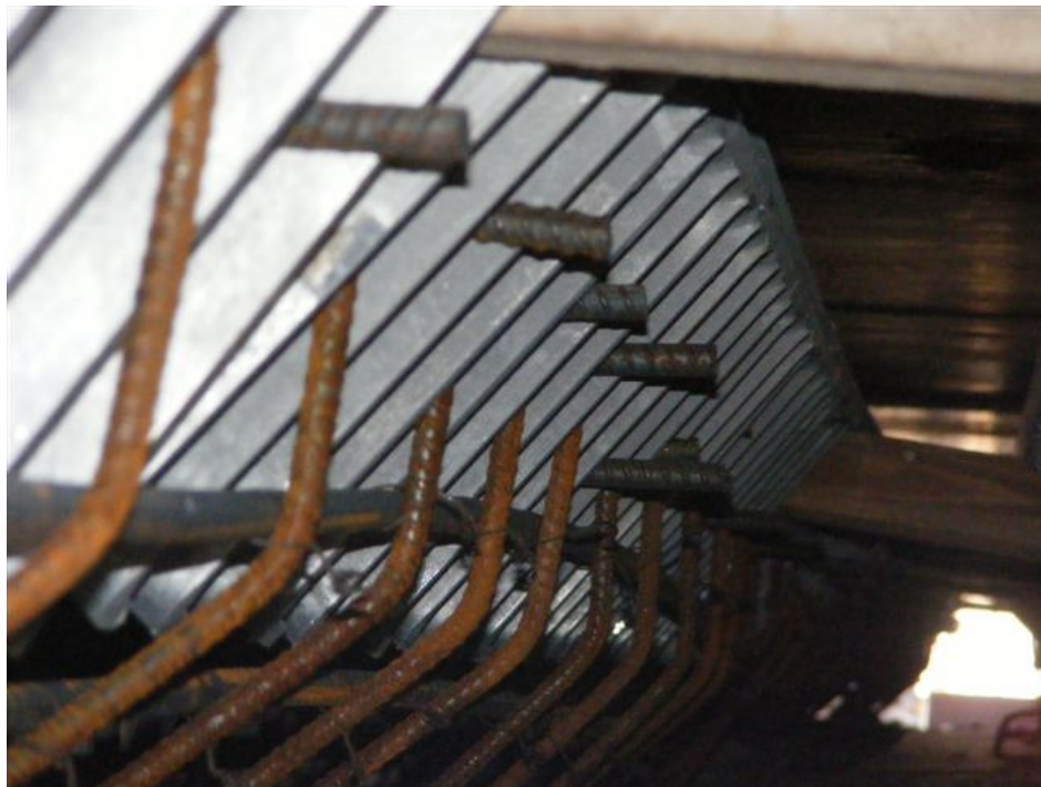
Fig. 16.12(B)-3 Photo of new Expansion device shown in Fig. 16.12(B)-2
