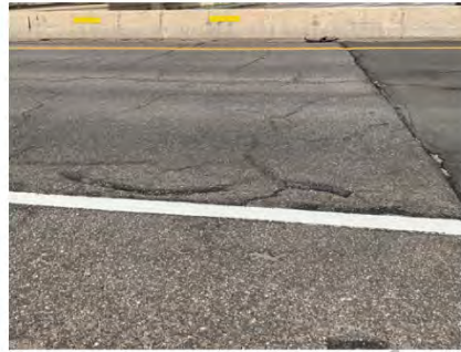
Span 4 has up to wide longitudinal and transverse cracks on asphalt some previously been sealed, but failed in spots.
