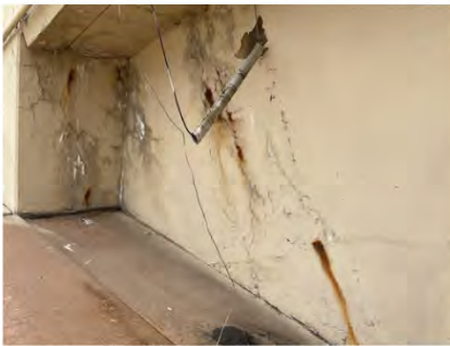
Abutment 5 backwall has a 0.016 inch wide diagonal crack with efflorescence and shrinkage cracks with rust stains below the Left overhang.
