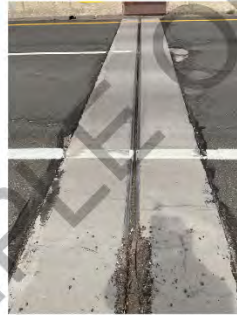
Forward joint glan is failed in mainlines.
