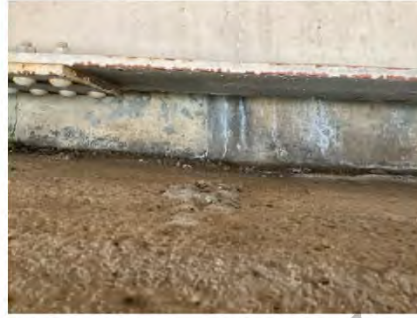
Some waterstains due to joint leakage at Abutment 1.
