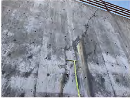
Diagonal crack in southwest wingwall
