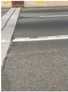
Pothole about 2 sq feet in center lane next to rear joint end dam.
