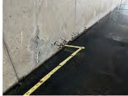
Honeycomb in bottom of Wall 2 Cell 1 near midpoint
