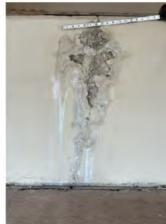
Abutment 5 has vertical crack with delamination and efflorescence at midway of breast wall.
