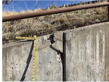
Spall in northwest wingwall
