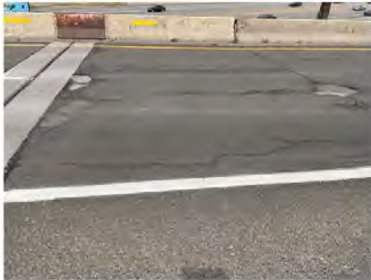
Abutment 5 has some longitudinal cracking and a 2 square foot pothole along the strip seal joint in Lane 2, and a pothole at the sleeper slab.
