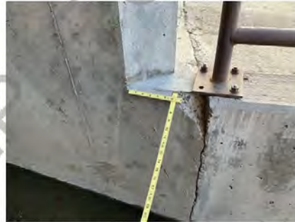
Spall in Wall 2 at inlet
