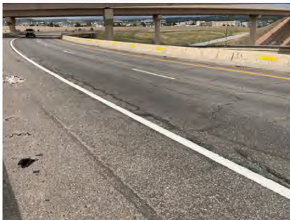
Span 4 has Wide longitudinal and transverse cracks in asphalt previously been sealed, but failed in spots
