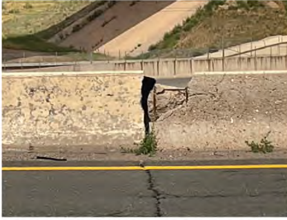
Forward Left Approach Rail has a spall with exposed rebar.
