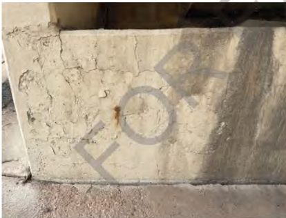
Abutment 5 has minor delamination around vertical cracks on the left side.
