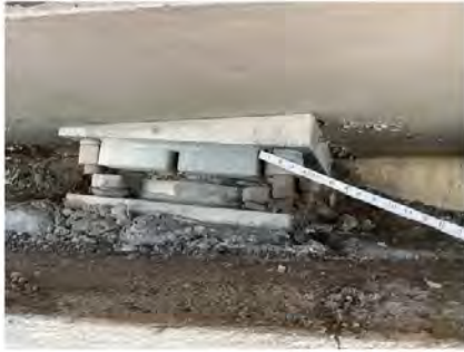
Sole plate and masonry plate anchors are in contact at Bearing 5A, the bearing is in the maximum expansion position, Bearing 5A is currently surrounded by debris,
