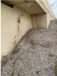
Random cracking with efflorescence and rust stains at Left of Abutment 1.
