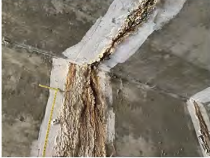
Heavy efflorescence buildup and rust staining in Wall 2 of Cell 2
