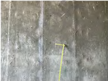
Vertical crack in Wall 1 near inlet
