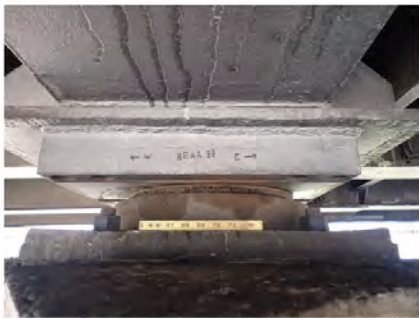
Limits of expansion and contraction for Bearing 3B 6/27/2025 12:00:00 AM
