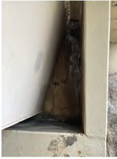
Abutment 1 has cracking with efflorescence and some rust stains at back wall, left side near Girder 1A .
