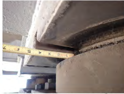
4.5 inches to edge of bearing plate on west side of Bearing 3B 6/27/2025 12:00:00 AM
