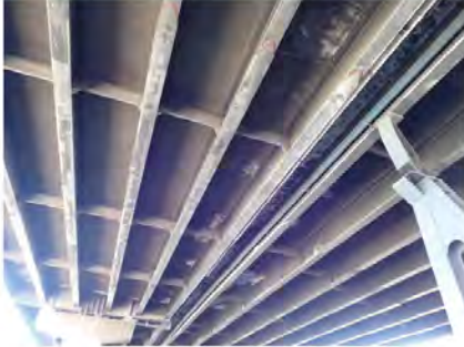
Efflorescence in deck soffit of Bay 3E
