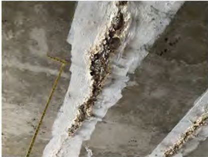
Rust staining and stalactites in bottom of top slab in Cell 2 near midpoint
