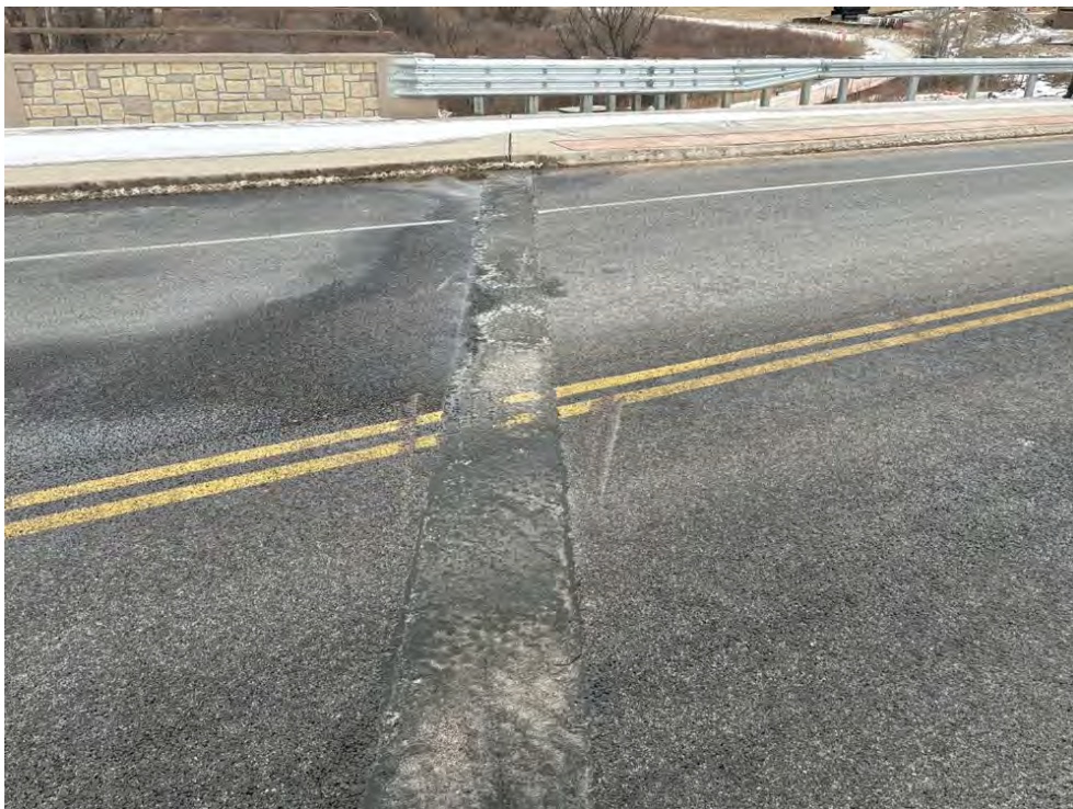
P - Plug (Rubberized asphalt/pourable)
