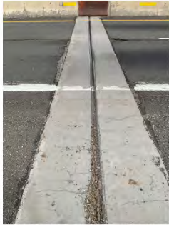
Abutment 1 joint is 38 feet long, it is open 1 inch and filled with sand in the shoulders.
