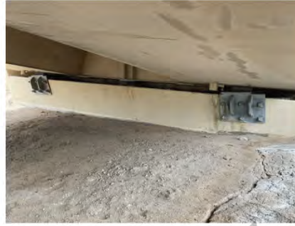
Abutment 1 up to medium width cracking
