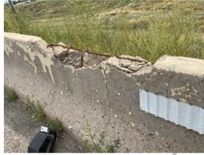
Forward Right Approach Rail has a spall with exposed corroded rebar,
