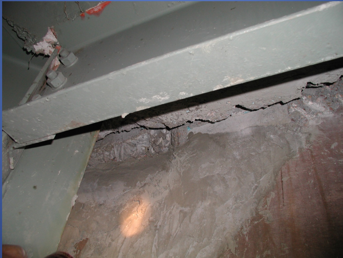
POOR CONCRETE CONSOLIDATION
