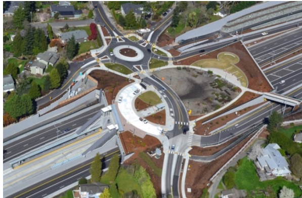
Granite’s recently completed SR-520 Project included a covered lid with urban landscaping.
