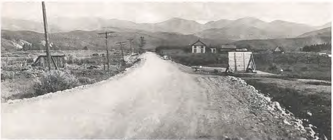
A fine stretch of Federal Aid highway looking east from Fraser, in Grand County, with James Peak in the distance.
