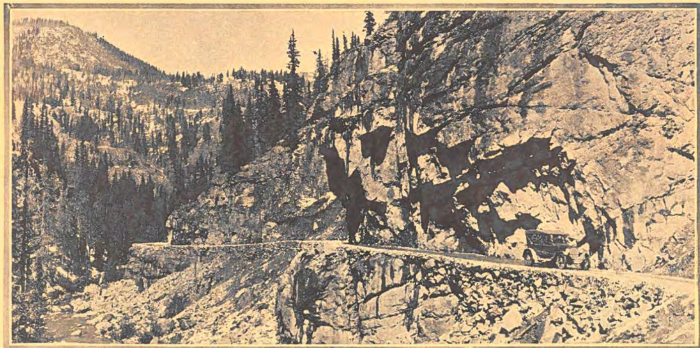
Wolf Creek Pass, on the state highway into Mesa Verde National Park via Durango. Here is where the road was blasted from granite.
