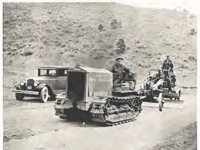
Another maintenance outfit employed by the state highway department on federal aid roads.
