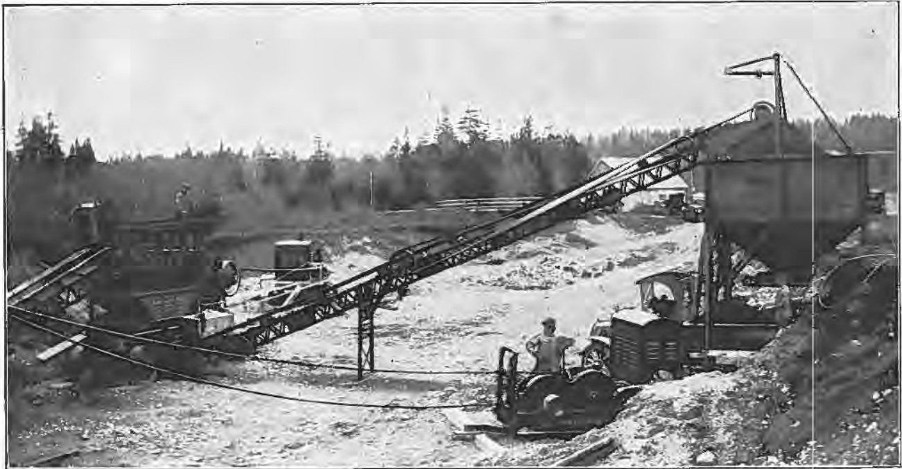
Pioneer Screening, Crushing and Loading Plant No. 10, sold to the Provincial Highway Board, Nova Scotia, Canada, by "Pioneer" Distributor, W. G. Stanfield of Sydney, N. S. Picture shows No. 10 Plant at left, with 55 ft. Steel Frame Loading Conveyor leading to 21-yard bin, at right.
