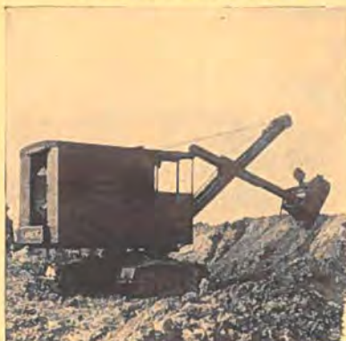
New economies in excavating. This compact outfit handles 500 yards in 10 hours, is easily and quickly moved in close quarters, and operates with remarkably low fuel consumption.
