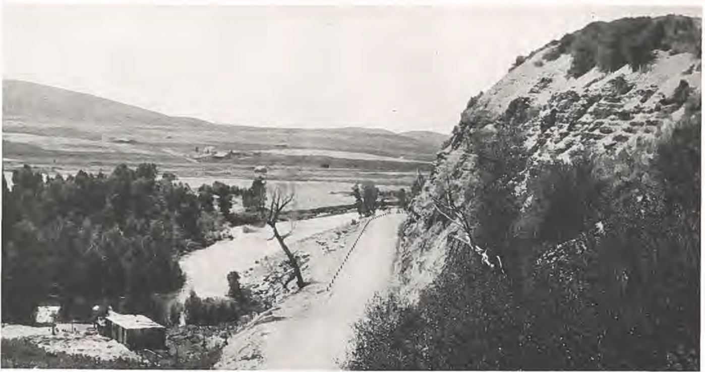
A section of completed road near Milner, west of Steamboat Springs on the Victory Highway—another State Highway Department achievement.
