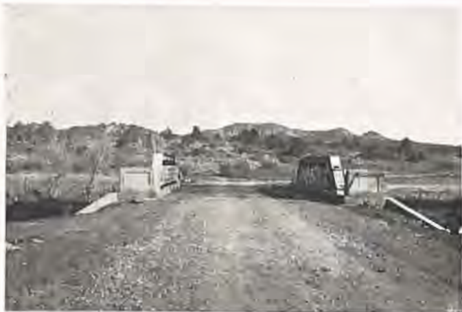
Newly completed gravel road and concrete bridge near Bondad in La Plata county.
