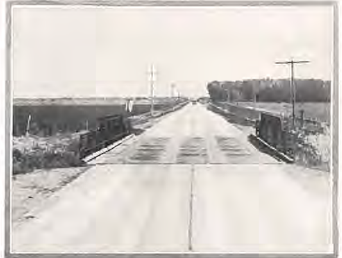
Showing stretch of newly completed pavement near Fort Morgan on U. S. Highway No. 38.
