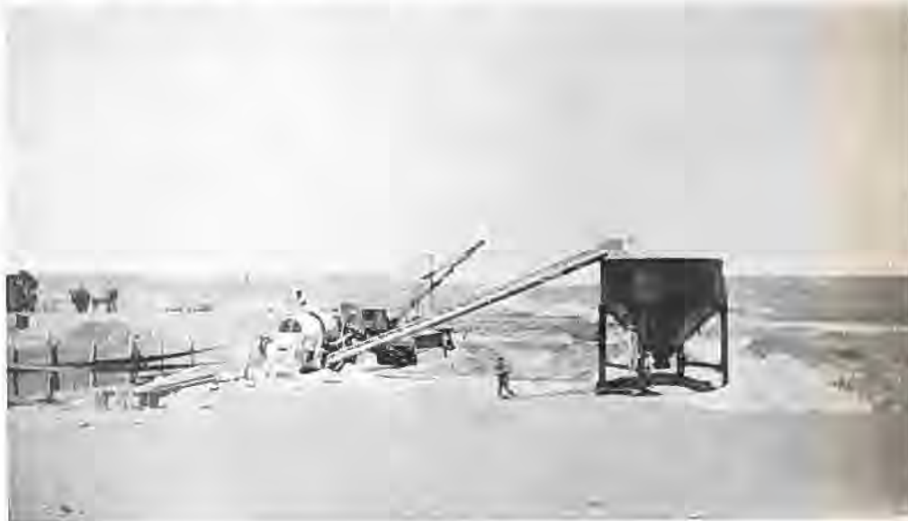
A portable screening and crushing plant used in preparing material for oil processing near Dover on State Road No. 1.
