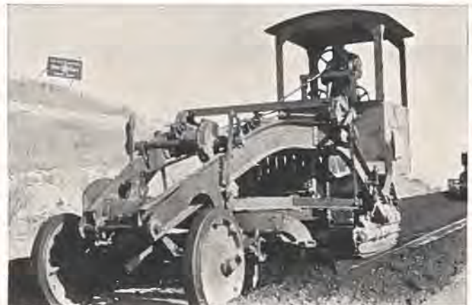
Showing Adams one-man maintainer "turning oil mix" on highway south of Cheyenne, on State Road No. 1.
