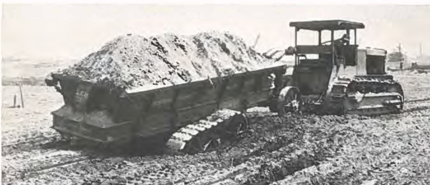
A Monarch tractor pulling a new type Western Crawler wagon, loaded to the "gun-wales"—another modern road construction unit.
