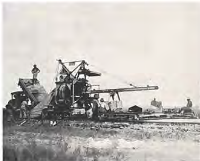
Concrete paver at work on Selander contract near Wiggins on U. S. Highway No. 38.
