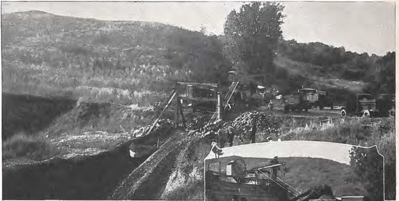
No. 12 Pioneer Screening, Crushing and Loading Plant hooked up with drag line and Caterpillar 60 H. P. unit, operating on regraveling job on section of Stillwater cutoff. Roth Construction Company of St. Paul, contractors and owners of this equipment.
