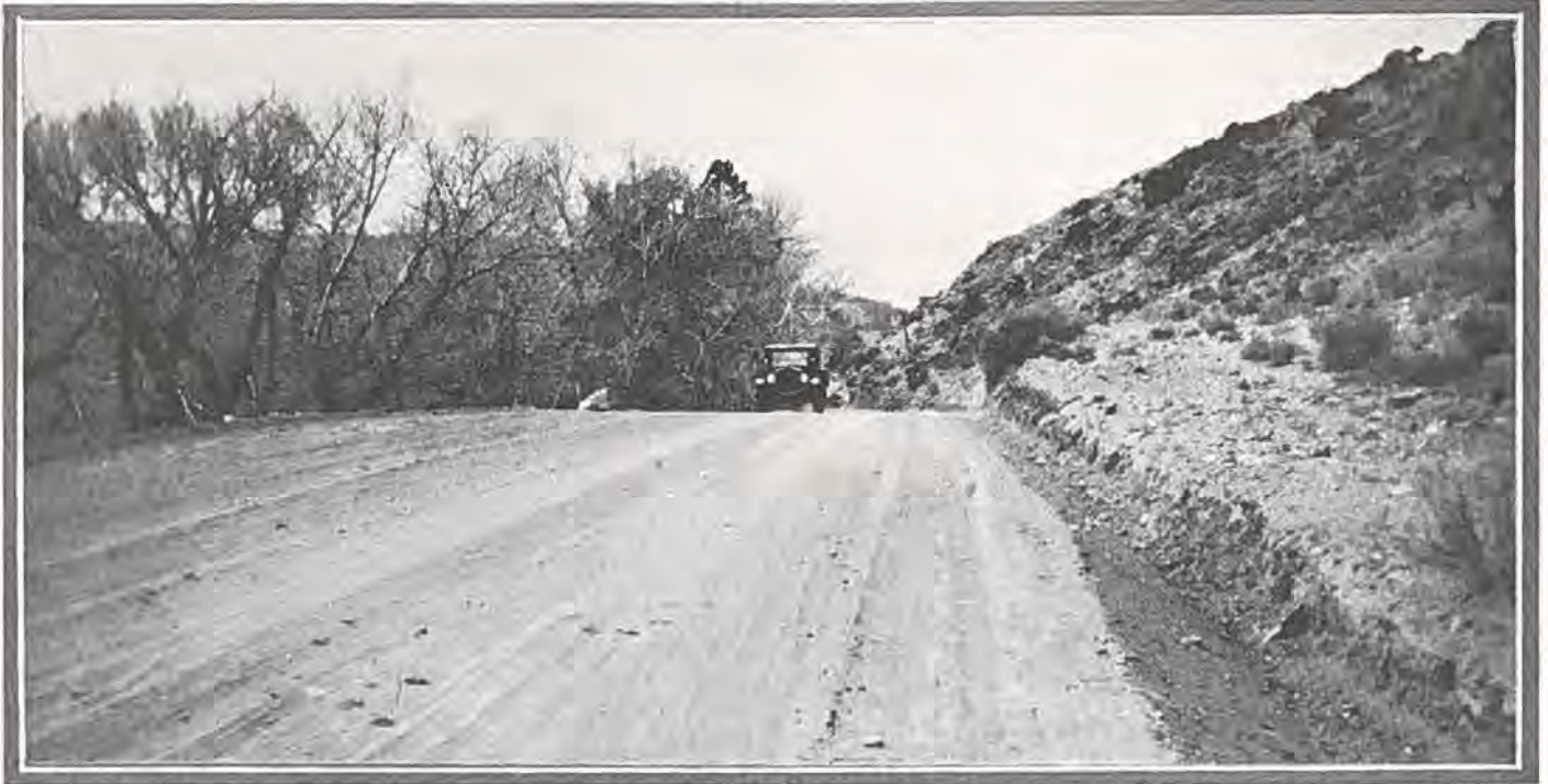
Showing a section of the La Veta Pass highway, maintained by state forces.
