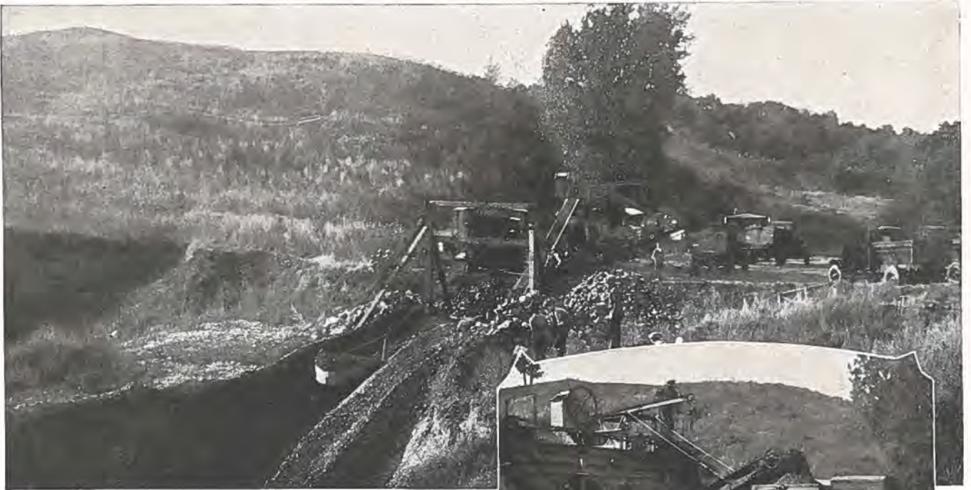
No. 12 Pioneer Screening, Crushing and Loading Plant hooked up with drag line and Caterpillar 60 H. P. unit, operating on regaveling job on section of Stillwater cutoff. Roth Construction Company of St. Paul, contractors and owners of this equipment.
