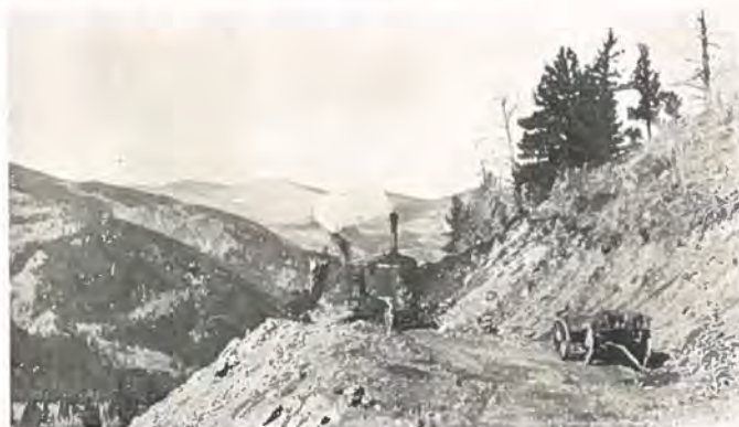
Steam shovel digging out the side of a mountain for the new highway.—Photographs furnished by U. S. Bureau of Public Roads.
