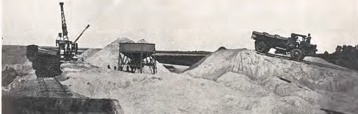
Showing method of handling sand and gravel by contractor on Fort Morgan paving project.
