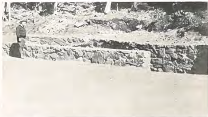
One of the many special culvert intakes constructed of rock and concrete on the Chicago Creek highway.
