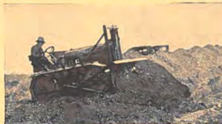
Backfilling sewer trenches in Milwaukee. This crawler-mounted McCormick-Deering puts back a great volume of dirt with ease and efficiency.
