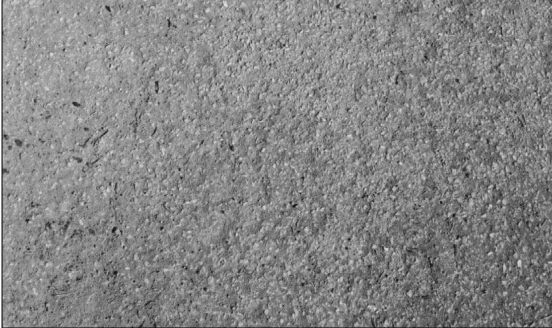
Plate 31. Worn asphalt. State Highway 13 (Main Street) in Meeker.
