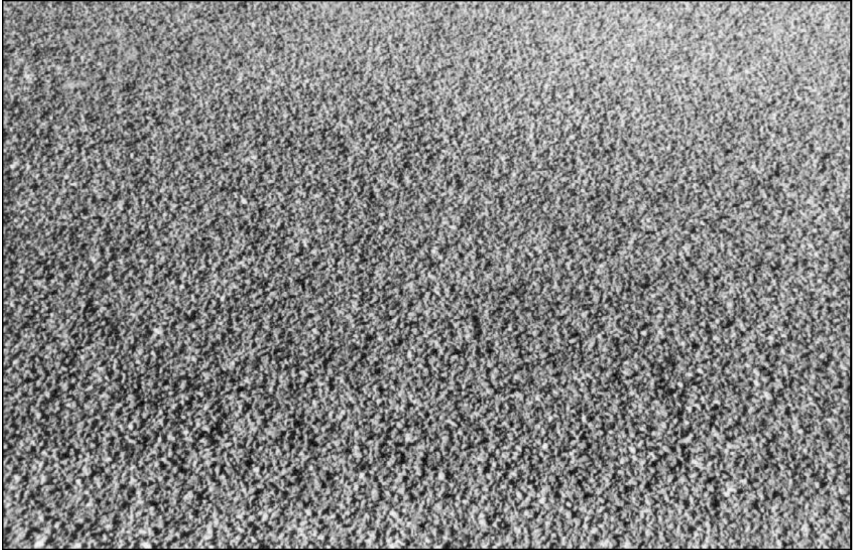
Plate 24. Large chunks of aggregate on old US 85; approximately 500 feet west of I-25.
