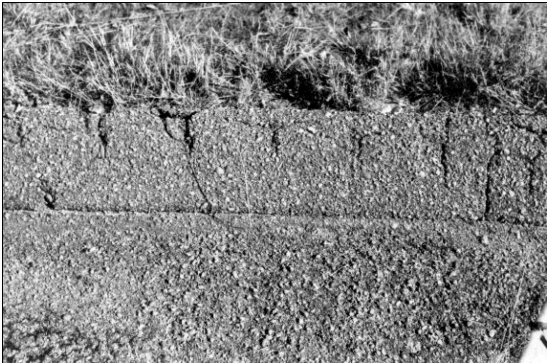
Plate 23. View east of curbing leading to drainpipe near South Platte River on US 6.
