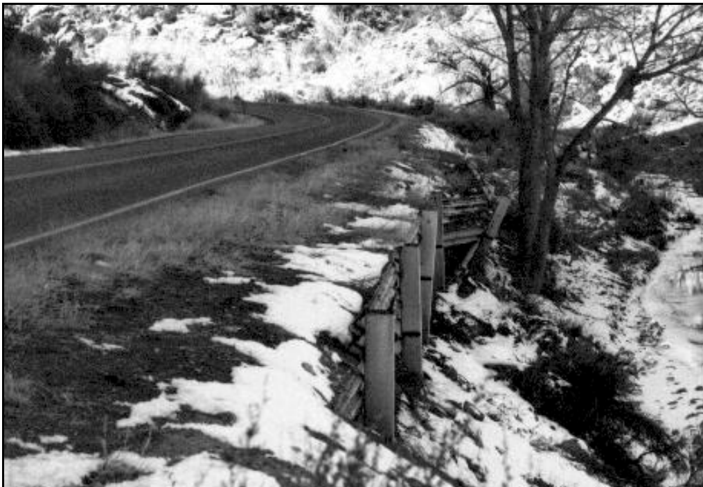
Plate 15. Eroded metal retaining wall above East Creek on SH 141.
