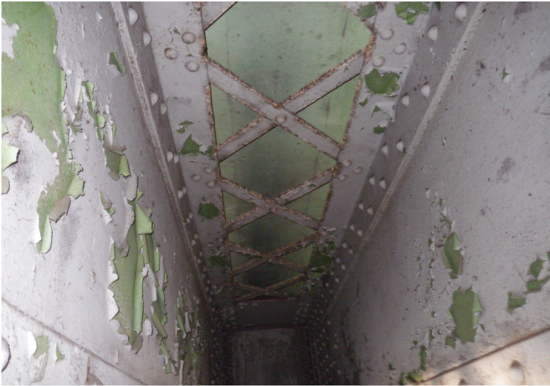
Figure 4.17. Heavy Metal-Based Paint Chipping
