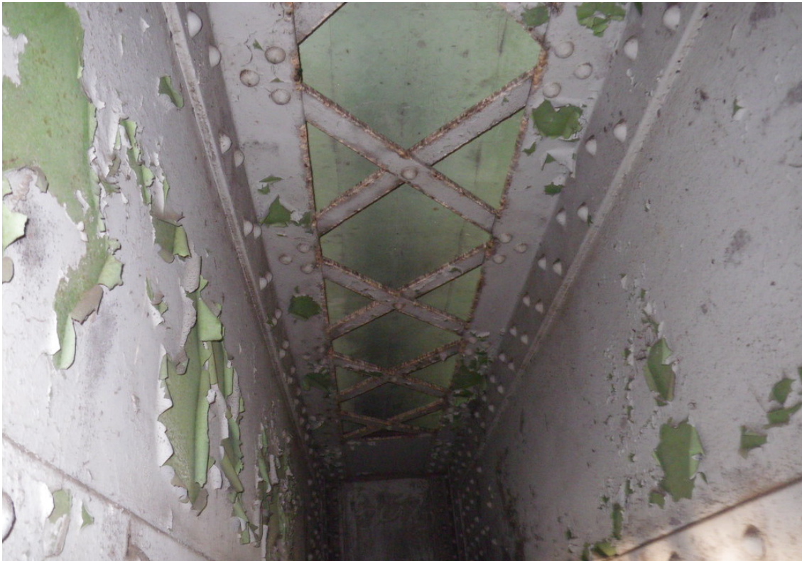
Figure 4.17. Heavy Metal-Based Paint Chipping
