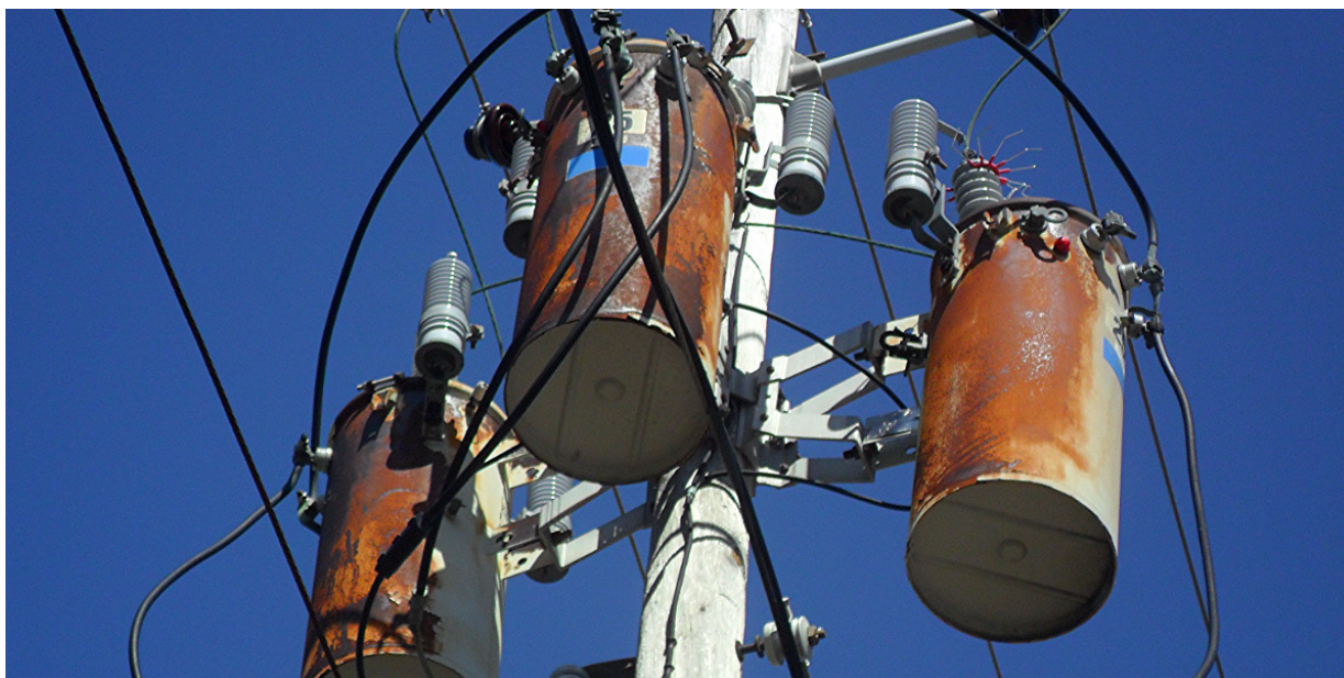
Figure 4.19. Three Pole-Mounted Transformers
