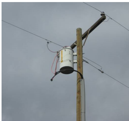
Pole-mounted electrical transformer in highway right-of-way.
