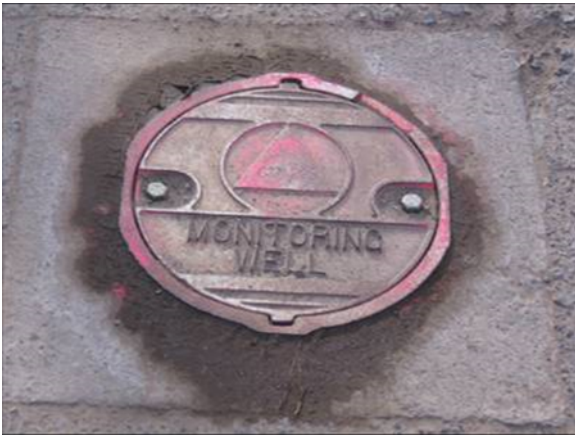
Flush-mount monitoring well.
