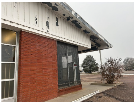
Chipping paint on a commercial property.
