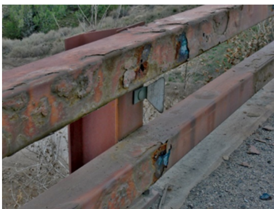
Chipping paint on a bridge rail may contain heavy metal-based paint
