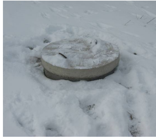
Likely residential septic system port.
