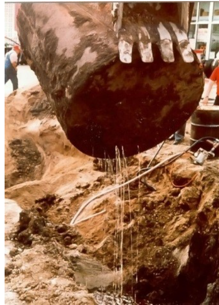
Figure 4.22. Steel Underground Storage Tank Leaking During Excavation
