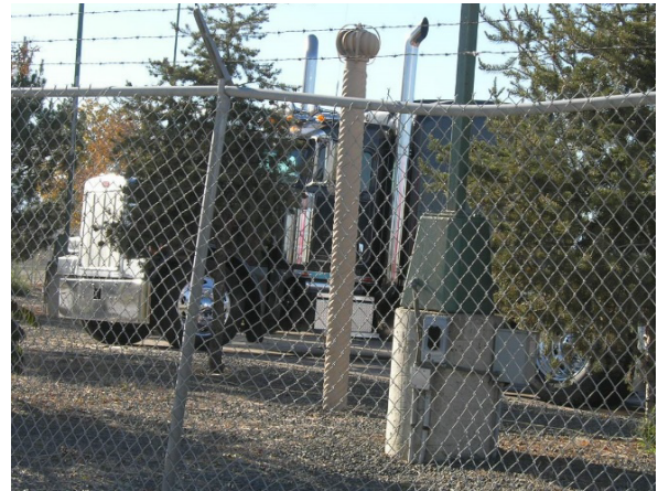
Vent pipe that may be connected to a former landfill beneath the ground surface.
