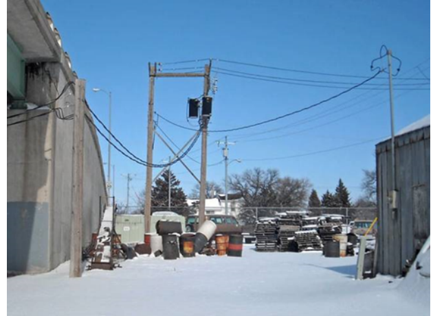
Pole-mounted electrical transformers. (Note drums in bottom half of picture).
