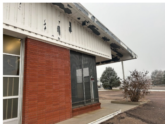
Chipping paint on a commercial property.
