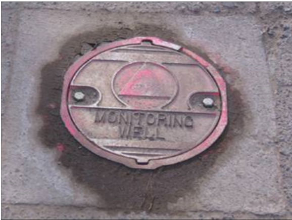
Flush-mount monitoring well.
