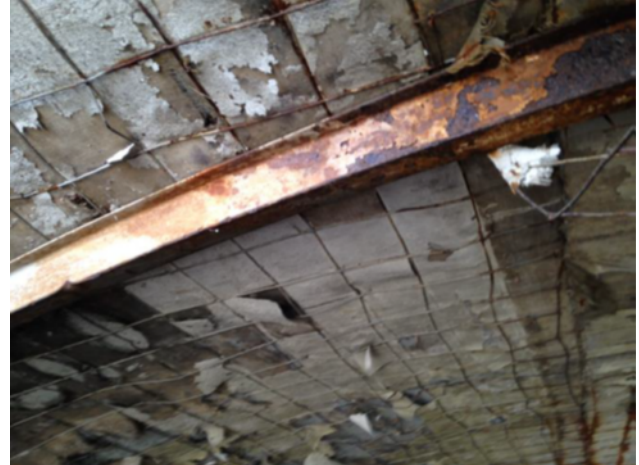
Potential ACM in fabric insulation inside a sand dome.
