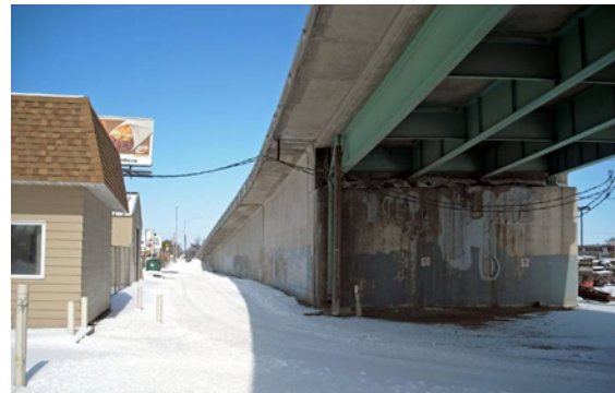
Paint on old bridges may contain heavy metal-based paint.
