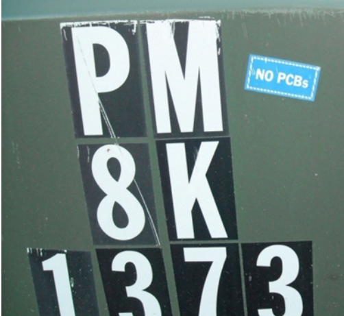
Pad-mounted electrical transformer with a No PCBs label.
