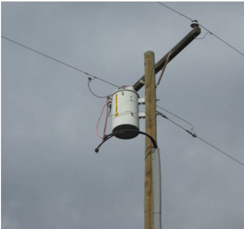
Pole-mounted electrical transformer in highway right-of-way.
