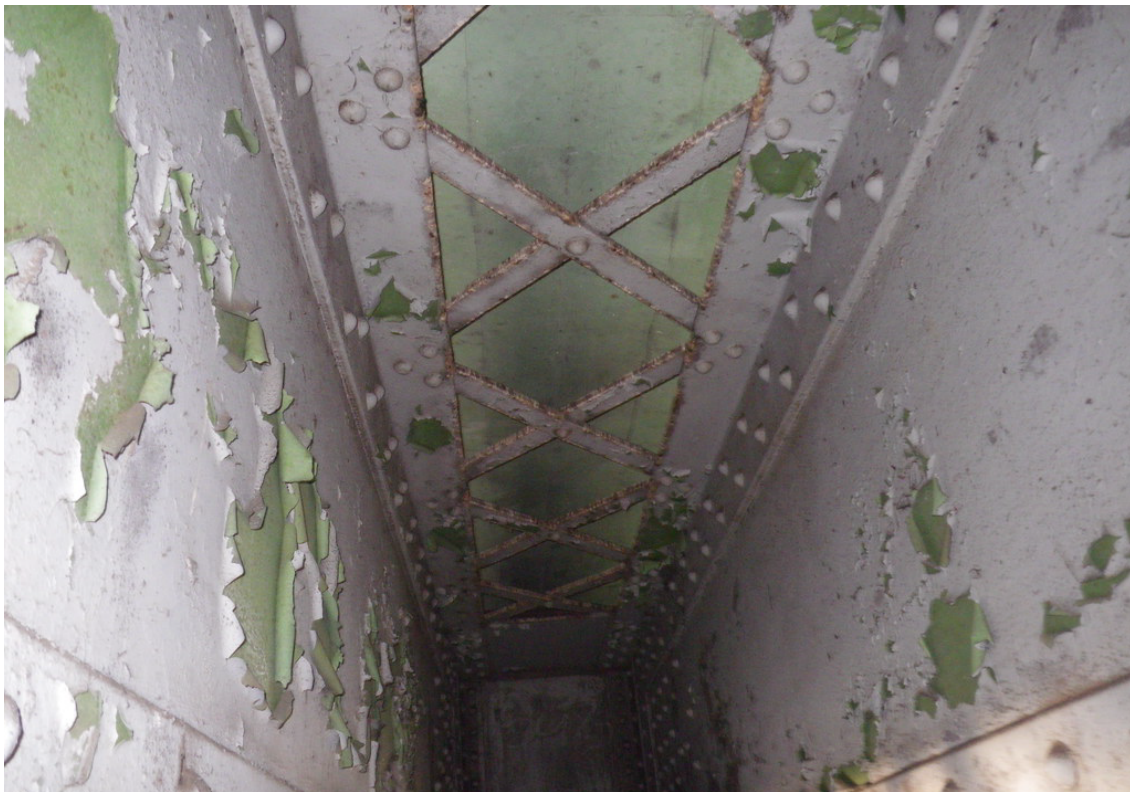
Figure 4.17. Heavy Metal-Based Paint Chipping
