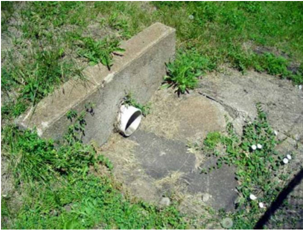
Drain pipe observed on the property of a foundry facility.
