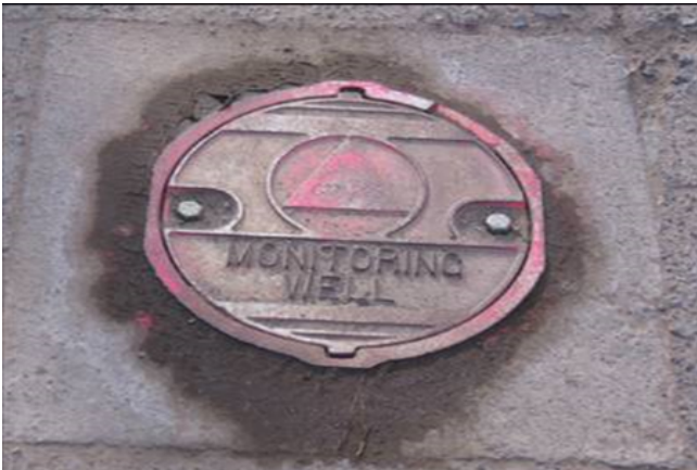
Typical in-ground monitoring well.
