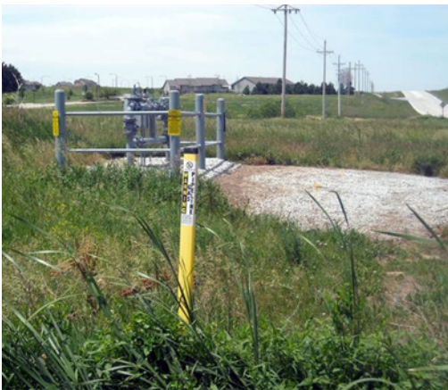
Gas line marker and regulator (background).
