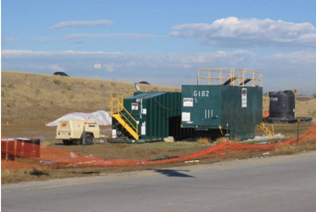
Baker remediation tank in highway right-of-way.
