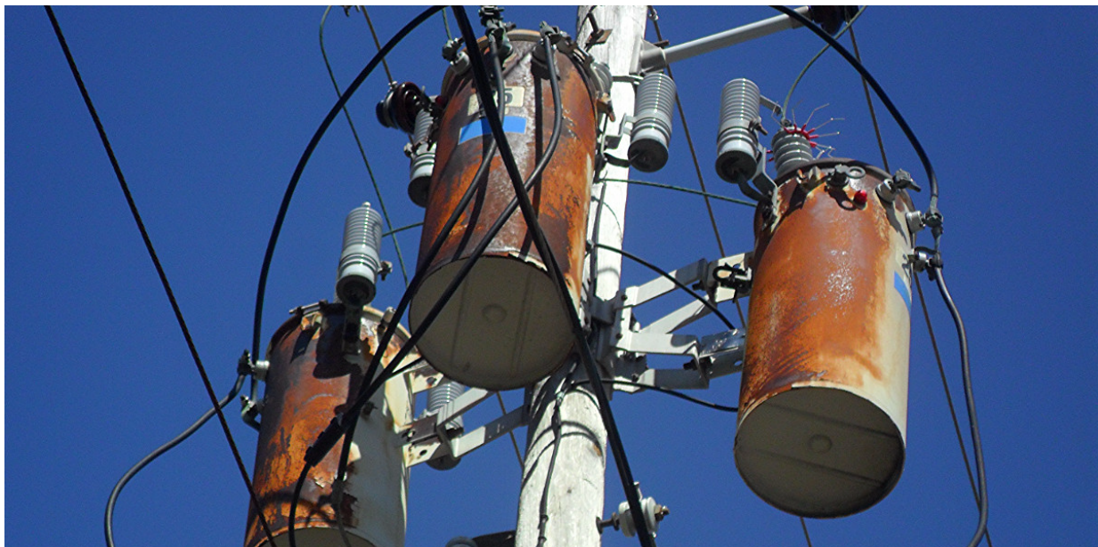
Figure 4.19. Three Pole-Mounted Transformers
