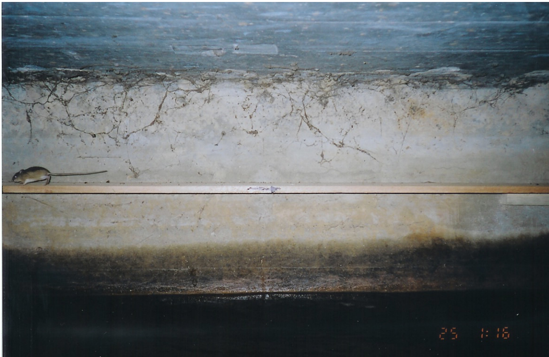
Photograph of a Preble's meadow jumping mouse using a ledge installed in a culvert under US36. Arrow indicated direction of water flow. Photo by Carron Meaney.
