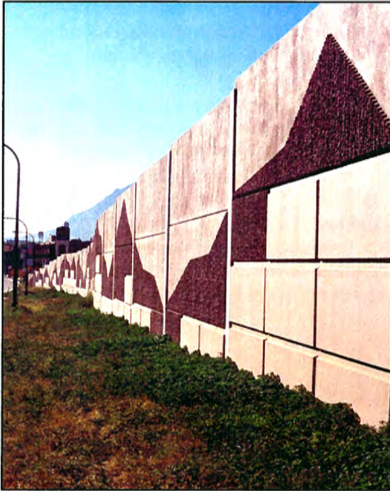
Figure 2-59. This noise wall is one of five that are found along Interstate 25 through Colorado Springs. Eight more are planned.
