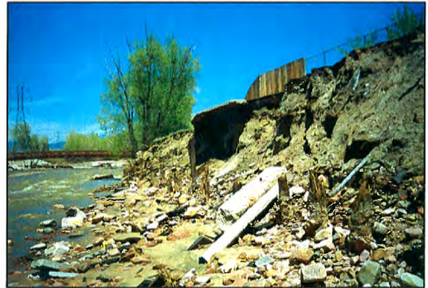
Figure 2-39. Flood damage on Fountain Creek Trail, Colorado Springs, 1999.
