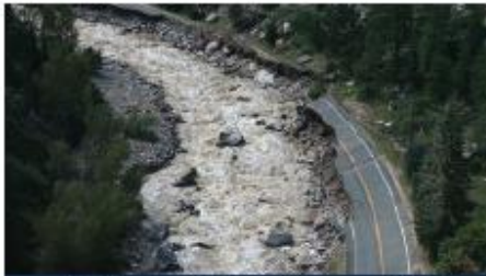
In September 2013, flood damage on US-34 destroyed an entire section of roadway.
