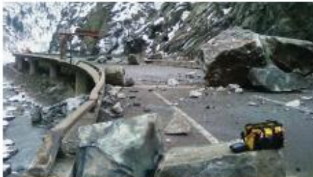
In February 2016, a rockfall closed I-70 in Glenwood Springs for two weeks.
