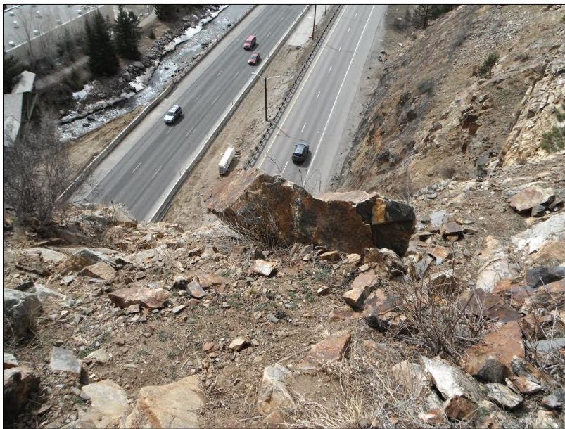
Figure 20. Rockfall Potential near Twin Tunnels on I-70
