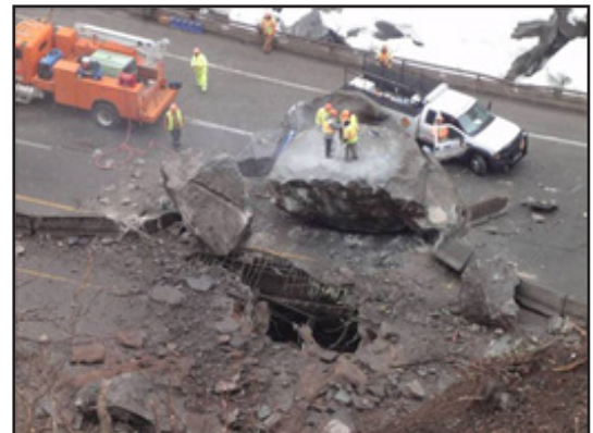
I-70 Glenwood Canyon Rockfall, 2016
