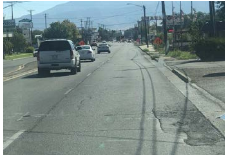
Poor pavement along a rural state highway.
