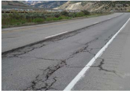
Pavement in need of repair along I-70.
