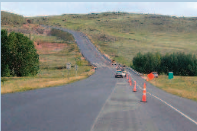
US 287 Virginia Dale north & south: resurfacing and bridge rehabilitation Region 4 Virginia Dale north and south, resurfacing
