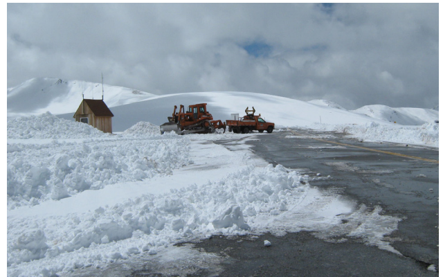
Crews worked around the clock to clear a late storm so SH 82 over Independence Pass could open by Memorial Day. [REGION 3]
