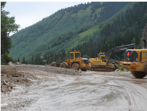
CDOT maintenance crews handle challenges brought on by Colorado's extreme weather, including mudslides like this one after an August rainstorm on US 550 north of Silverton. [REGION 5].
