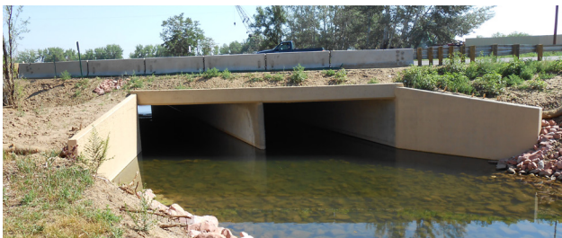
Dry Creek Bridge on US 287 in Ft. Collins was replaced with a concrete box culvert to meet new safety standards. [REGION 4]
