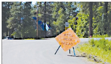
The need for proper construction zone signing
