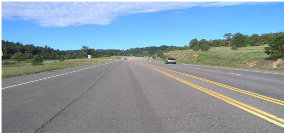
Figure 3. Looking south in the northbound lane ON us 285 at MP 224
