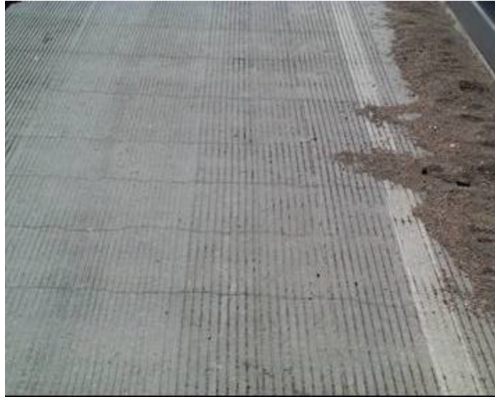
Figure F.2 Crack pattern at the end span (2.5 ft spacing)
