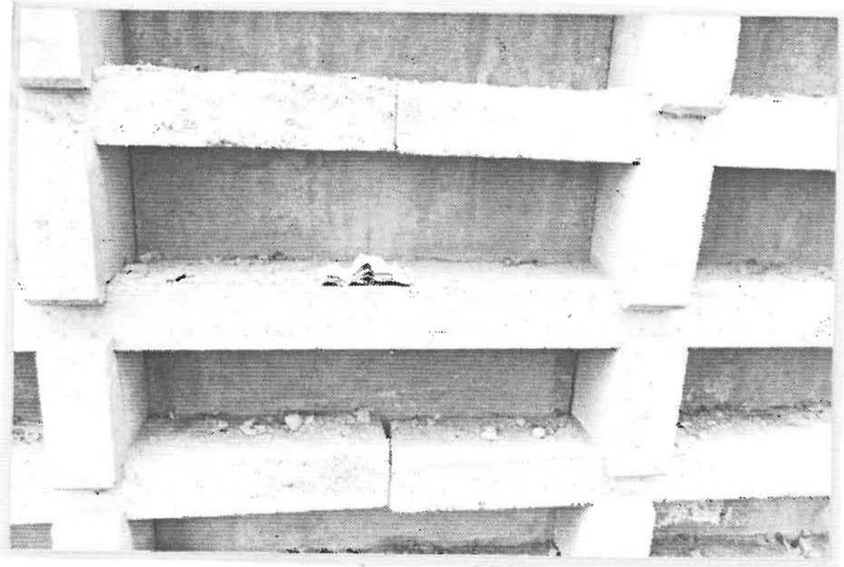
Figure 18 separation of the concrete blocks due to settlement of the foundation soils
