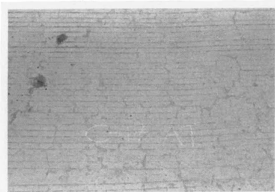
Photograph 9. Hairline cracks in deck. Structure C-17-AT. April, 1990. Low slump with fly ash.
