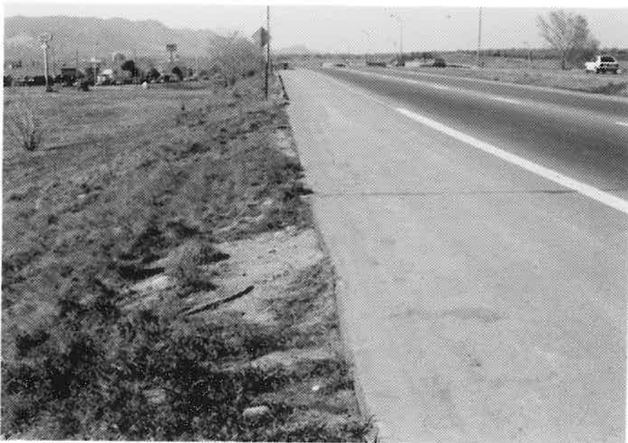
Photo 8. 3/16/87 I25 southbound, milepost 138, Harrison Road Interchange, 1986 epoxy paint.
