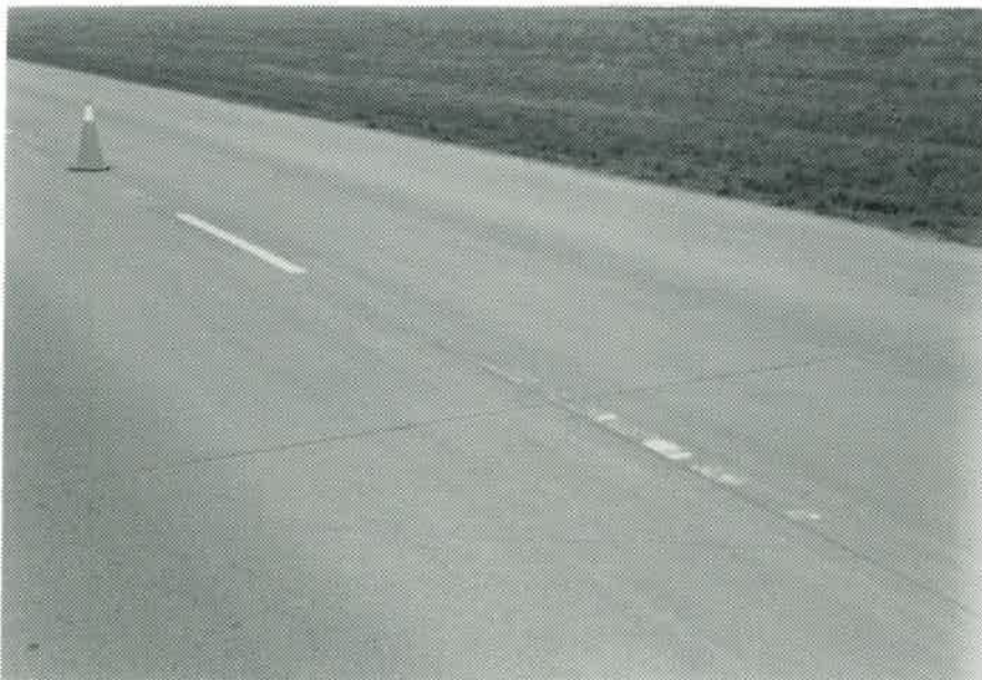
Photo 18. 2/27/89 I25 southbound, milepost 260 near Fossil Creek, 1986 extruded thermoplastic skip stripe on lower right and 1988 epoxy paint skip stripe in upper left.
