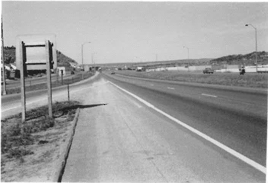
Photo 5. 3/16/87 I25 southbound, milepost 146, just north of Garden of The Gods Road, 1985 epoxy paint.
