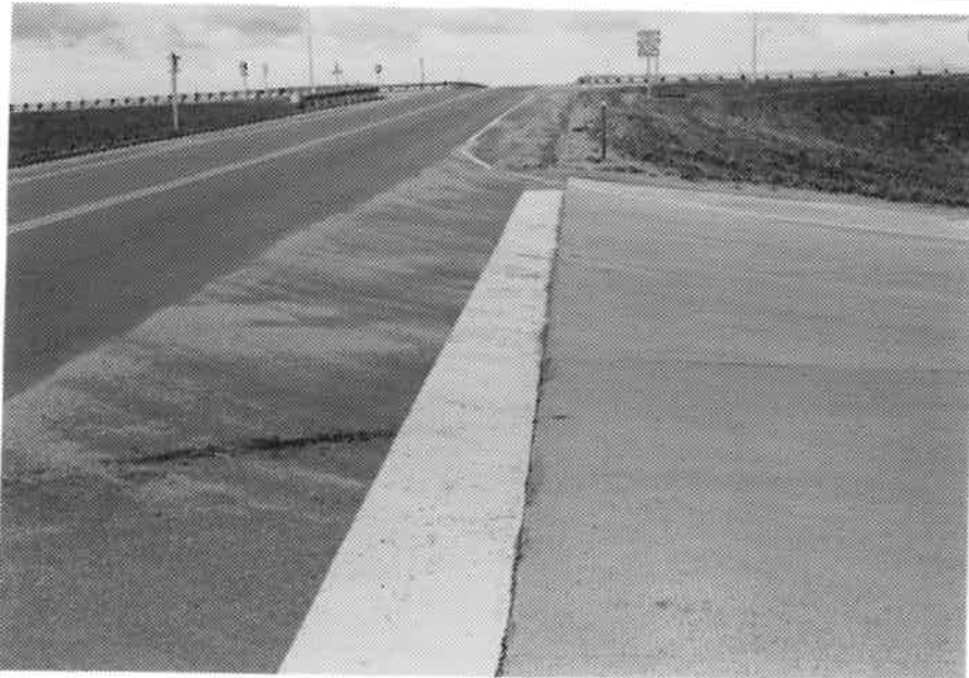
Photo 11. 4/13/87 Bromley Lane westbound, just east of I76, 1986 epoxy paint.
