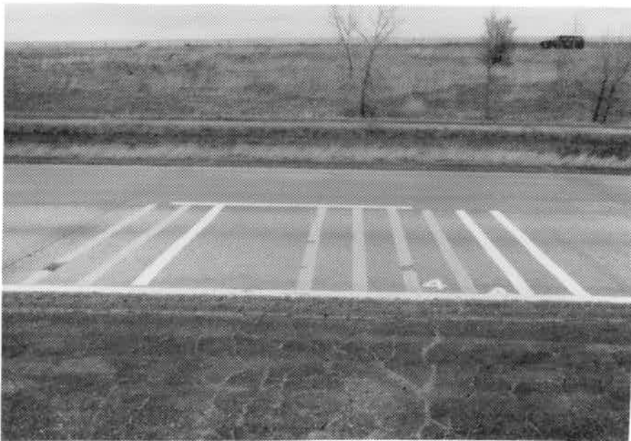
Photo 21. 3/29/88 Cataphote removable grade preformed plastic on concrete.
