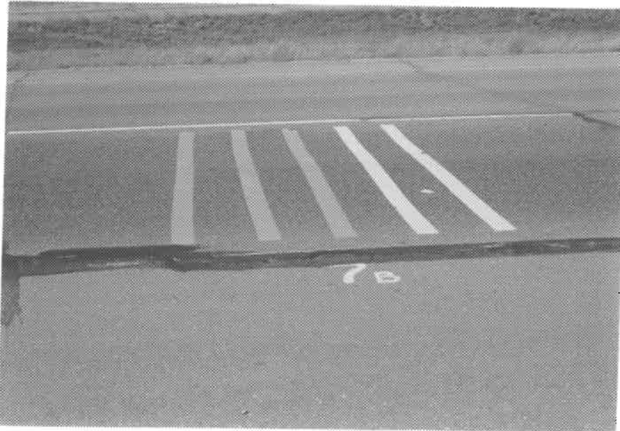
Photo 47. 3/8/89 3M0350 permanent grade preformed plastic on asphalt.
