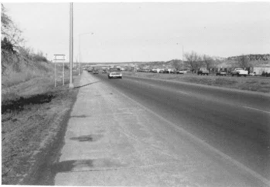
Photo 6. 1/25/88 I25 southbound, milepost 145, 1985 epoxy paint.
