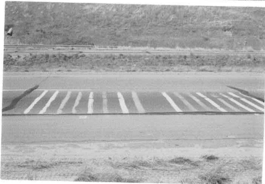
Photo 51. 3/8/89 Paints on asphalt.
