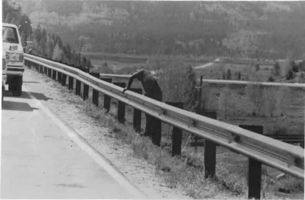
Photo A3. 10-gauge corrosion resistant guardrail with view of Camp Hale in the background.
