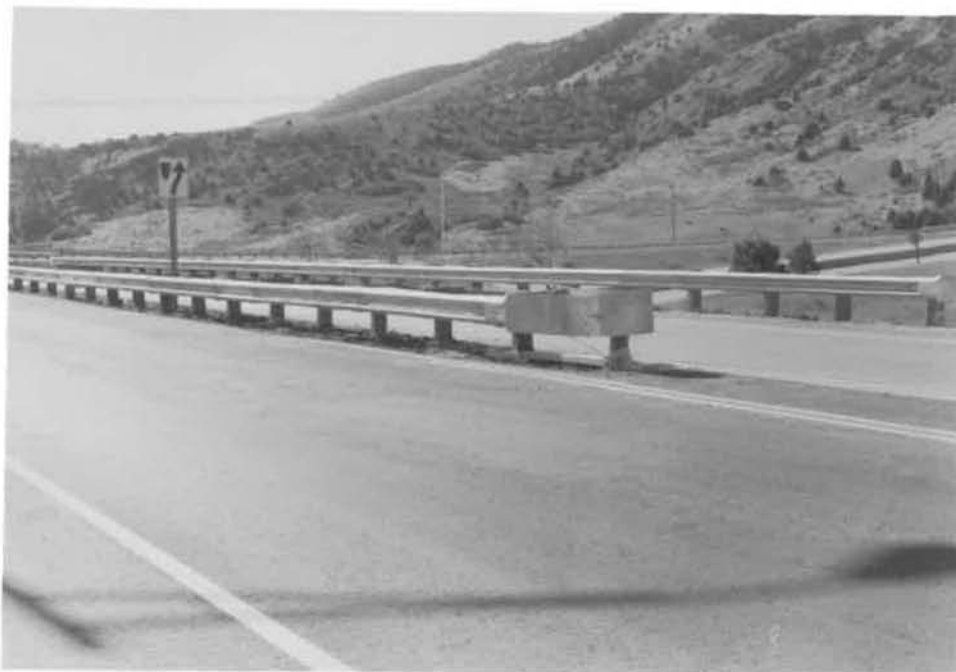
Photo C3. Side view of Crash-Cushion Attenuating Terminal (CAT) system.
