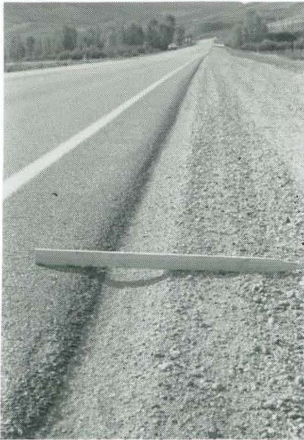
Photo 8 - Approximately 1 inch of rutting has occurred directly off the pavement within 3 weeks of maintenance work on the area.
