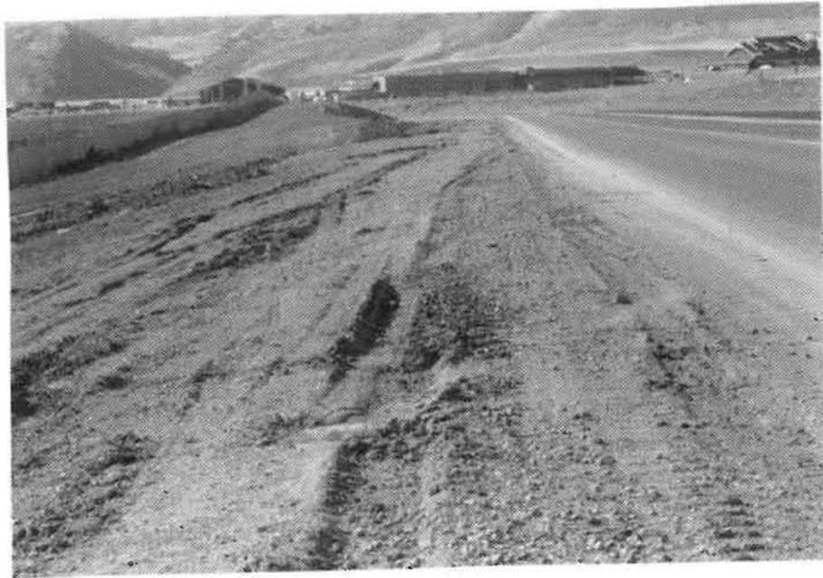
Photo 3 - This photograph and the next two show soft sections in the shoulder. The soft areas were caused by moisture.
