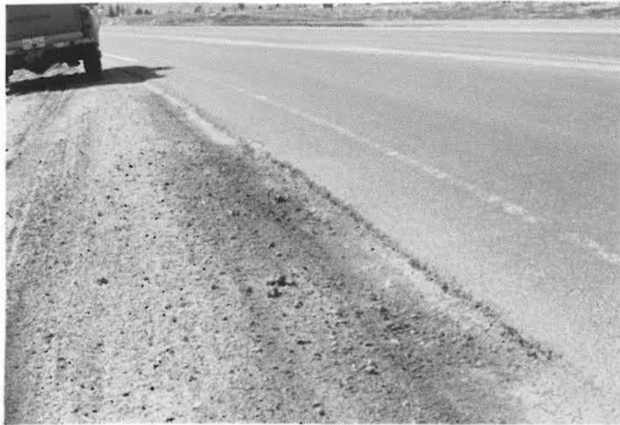
Photo 6 - This photo shows an area on S.Kipling where the pavement edge is spalling at the point where the gravel shoulder has been eroded away by vehicle traffic.
