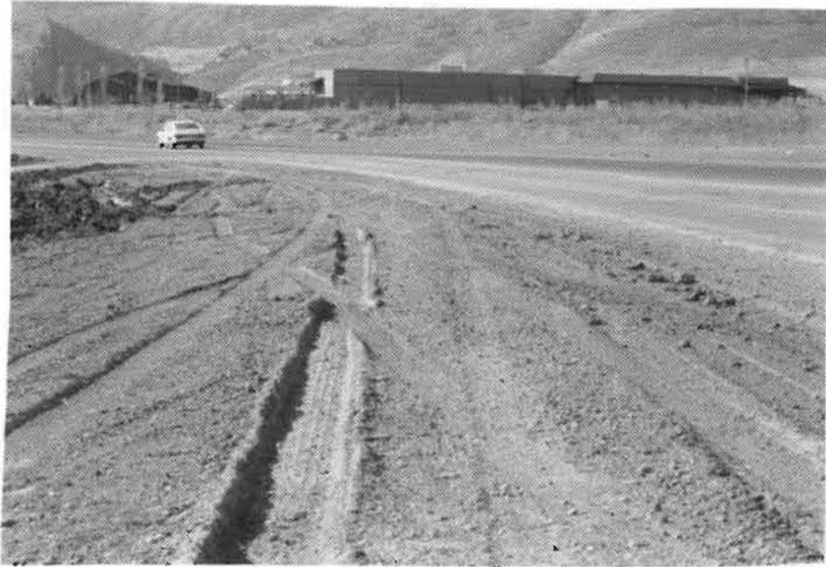
Photo 5 - Another soft area on the S.Kipling gravel shoulder.
