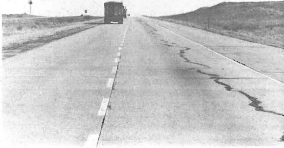
Trucks on I 76 use the passing lane to slow deterioration of the right driving lane.
