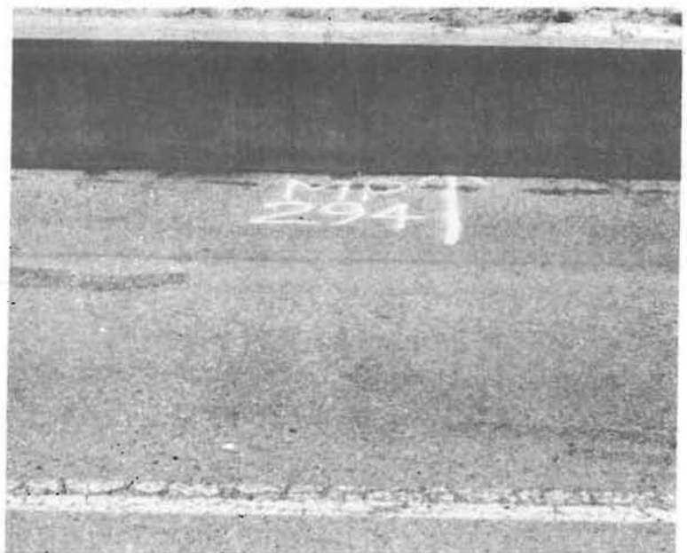
These are before and after photos of a hot in-place recycling project on US 50 near Penrose.
