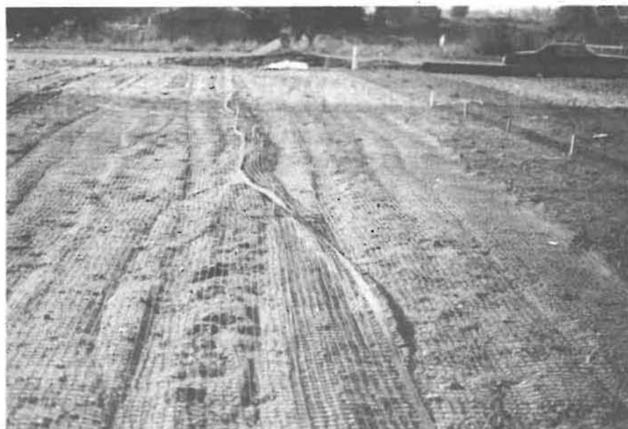
This geotextile is being laid to reinforce a 30-foot high embankment on top of a sanitary landfill filled with uniform fly ash.
