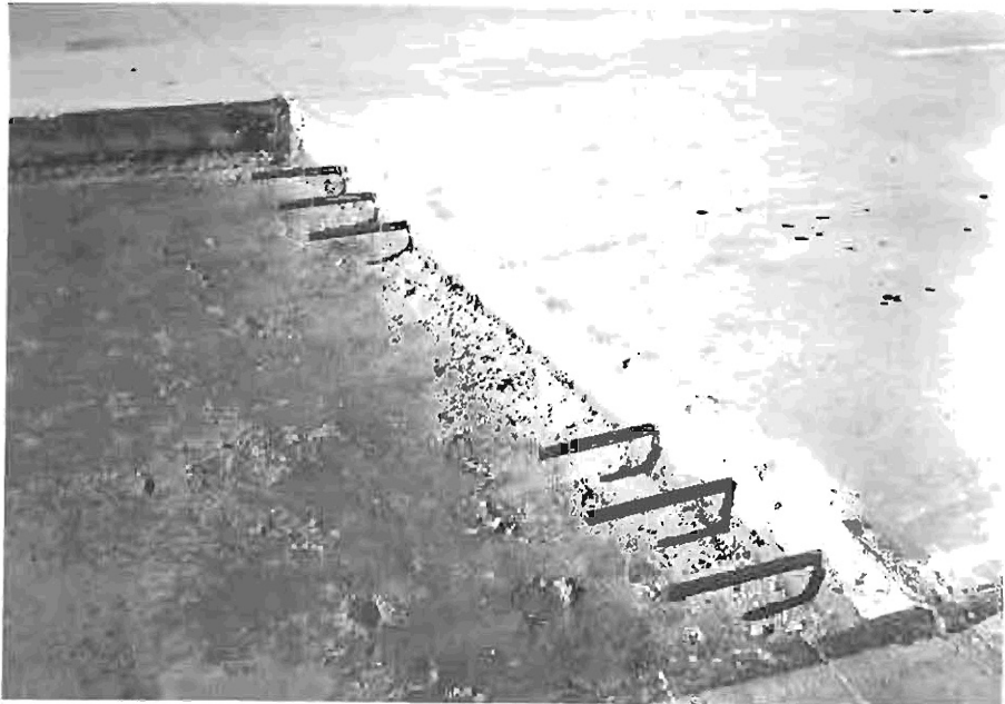
Photo 2: Insertion of dowels - three in each wheel path to improve load transfer for the replaced slabs.
