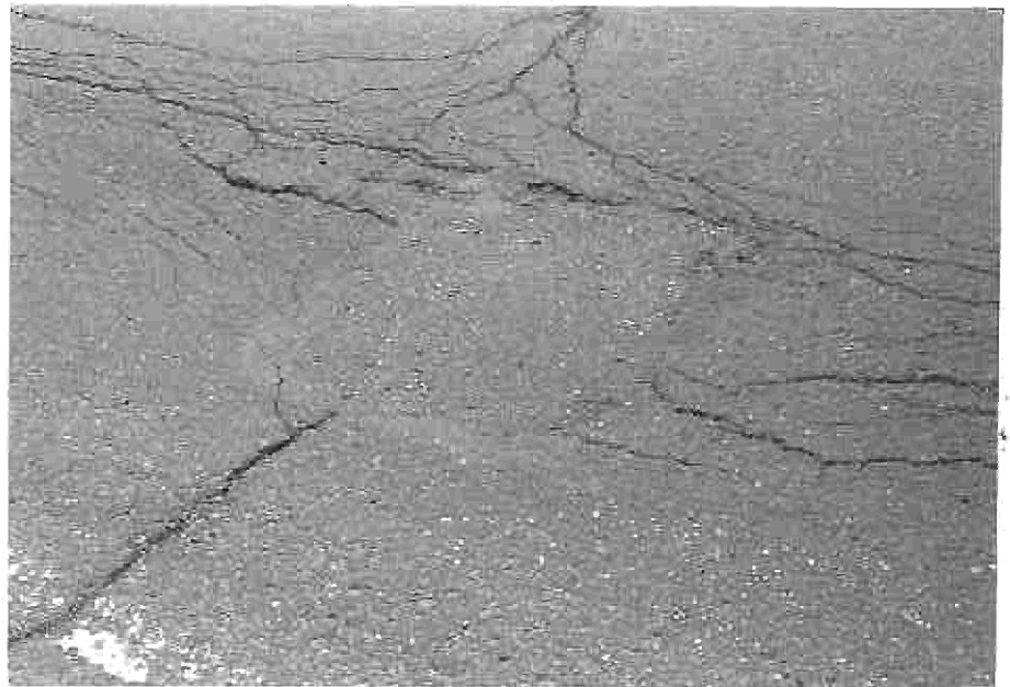
FIG. 12 After thirteen months the patch is solid. There is no separation around the edges and the alligator cracking around it has not damaged the patch.
