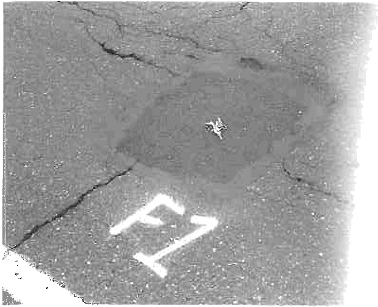
FIG. 11 The MC-250 with fibers patch is tight around the edges and shows no signs of problems after three months.
