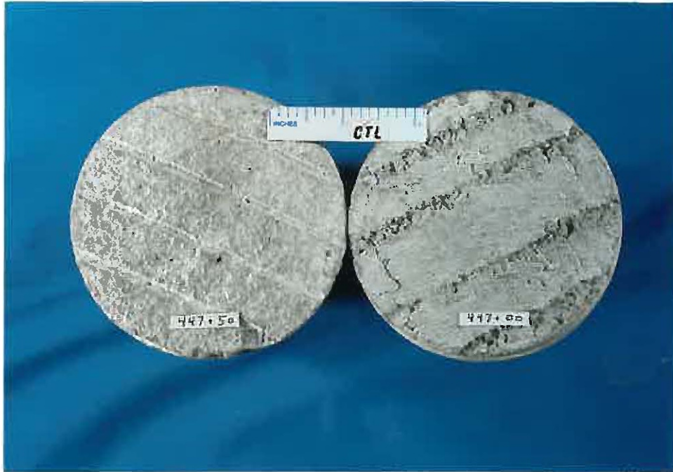
FIG. 1 TOP VIEWS OF CORE NO. 1 (447+50) AND CORE NO. 2 (447+00).
