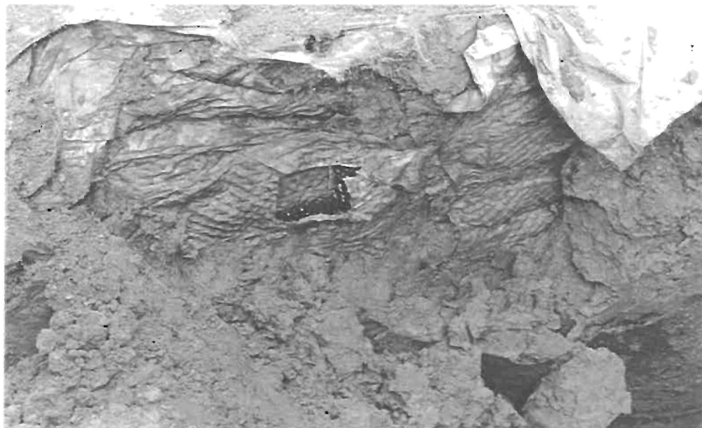
Figure 23 A piece of the curtain drain was cut out for further examination.
