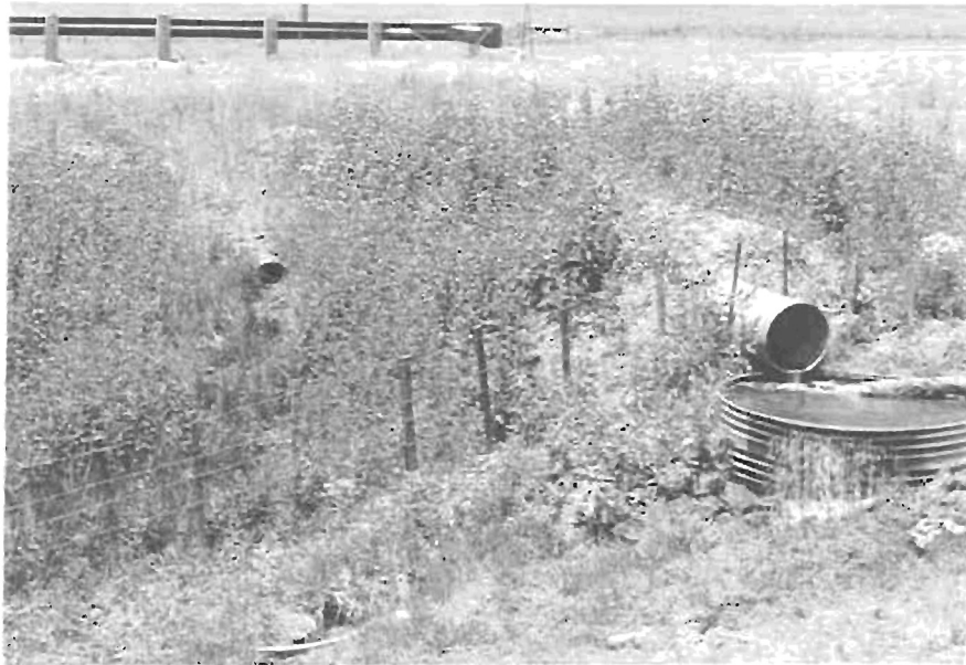
Figure 21. The culvert feeding into the tank on the right is bringing water from the ditch at the top of the slope on the other side of the roadway. The culvert to the left carries water from part of the southern section of curtain drain. This culvert is carrying very little water.
