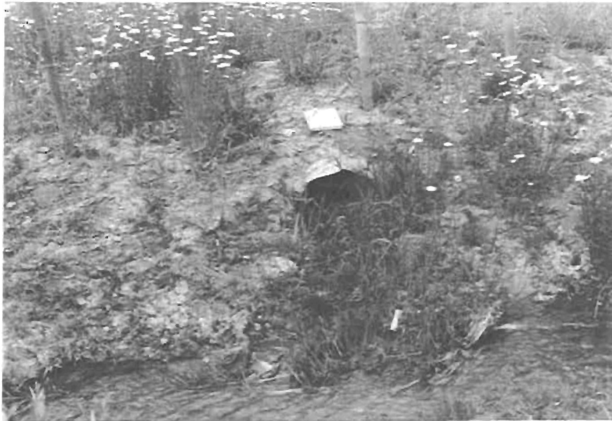
Figure 20 A relatively small amount of water, as seen coming from this pipe on the east side of the roadway, was collected by the system. The most observed was about 20 liters (5.3 gallons) per minute. The water in the foreground is from the roadside ditches and the channel above the curtain drain.
