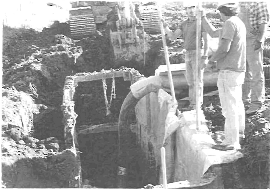
Figure 3 On the north side of this project it was necessary to use a trench box to keep the moisture saturated walls of the trench from collapsing. In this photo, the installation operation is progressing away from the camera. The perforated pipe is being fed through the bottom of the next drain section. When the leading backhoe pulls the trenchbox forward, the men on the right side of the photo will use the sticks with hooks to lower the drain sections under the brace and pull them back into place.
