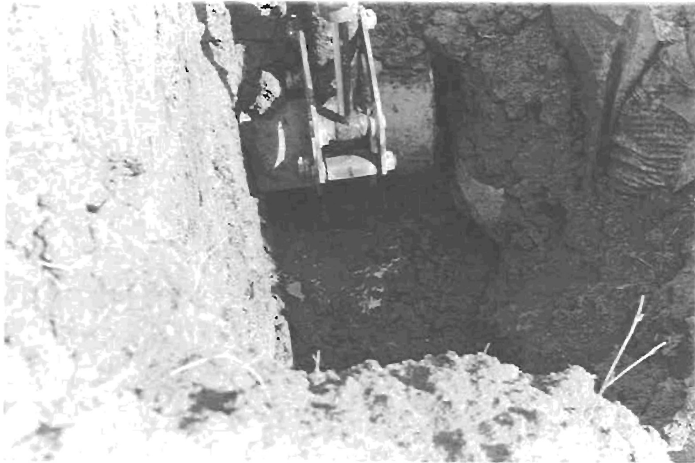
Figure 22 In September of 1990, a section of the drain was excavated with a backhoe and examined. The top of the curtain drain was found at a depth of almost two meters (six feet). The water in this photo at the bottom of the trench is due to the accidental cutting into the perforated pipe.
