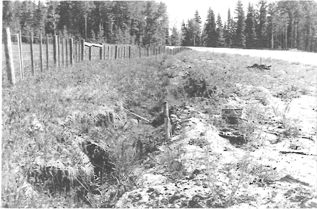
Figure 15 This moisture tube is adjacent to the interceptor ditch on the uphill side of the curtain drain.
