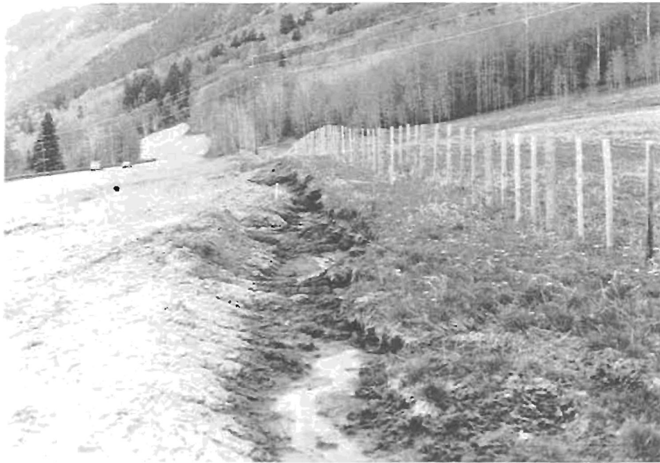
Figure 9 After the curtain drain was installed, it became apparent that there was a need to collect surface runoff as well. This ditch was dug at the top of the hill next to the right-of-way fence. The water was channeled to the roadside ditch.
