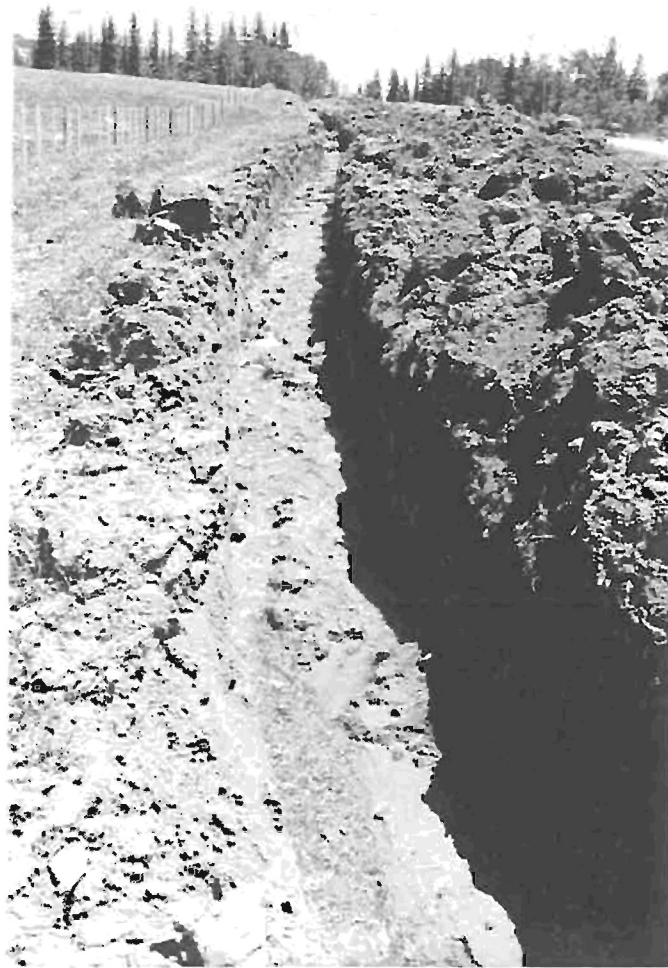
Figure 3 This is the initial phase of trenching at station 431+73 to 438+75. A stream of water can be seen flowing in the bottom of the trench.
