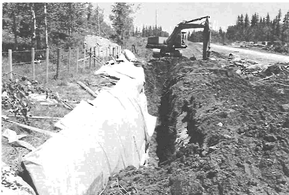
Figure 4 Pictured here is the installation on the south end of the project. The trench was dug in relatively dry soil which made it easy to hang the curtain drain sections from the fence, place them neatly and backfill the trench.
