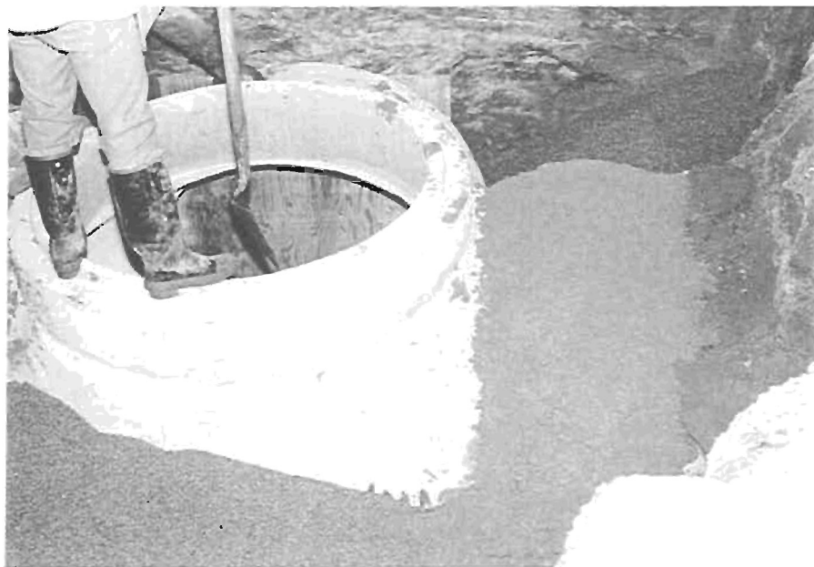
Photo 14 - The contractor used a class 2 backfill material around the manhole. By using this material the contractor was not required to use any devices for compaction.
