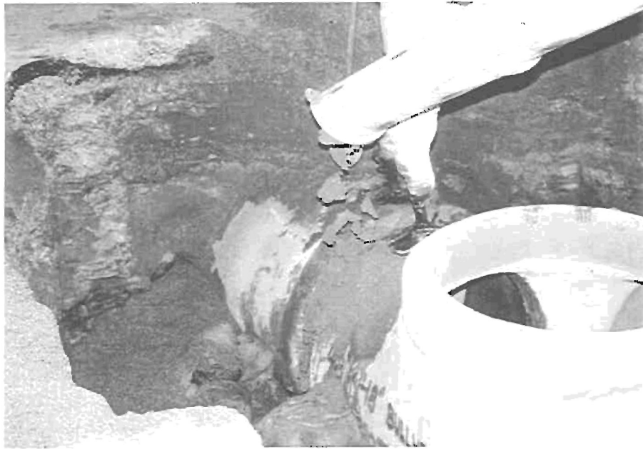
Photo 13 - Concrete with a 1-inch slump was used around the joint as a seal.
