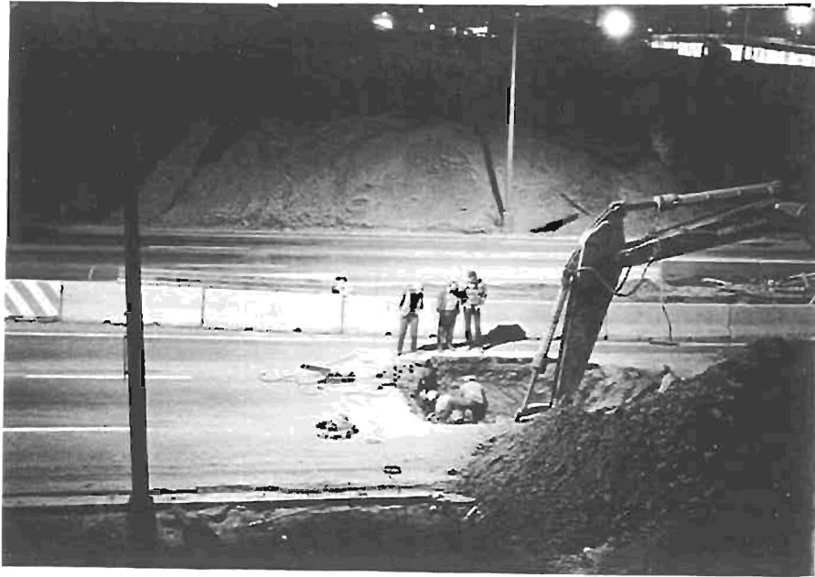
Photo 3 - Eastbound lanes on Hampden Blvd. were closed due to place the manhole. Excavation of existing storm drain required the entire width of roadway.
