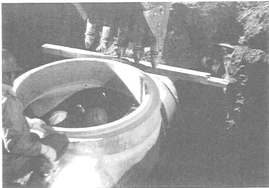
Photo 12 - After setting the manhole down a back-hoe was used to shift it vertically into position.
