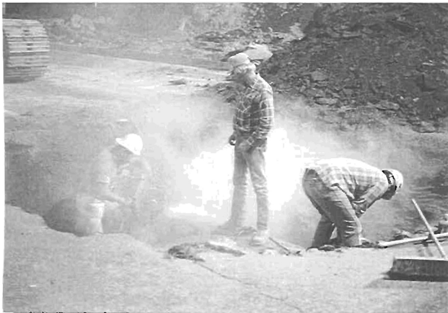
Photo 4 - A concrete saw was used to cut existing pipe allowing area for placement of new manhole.
