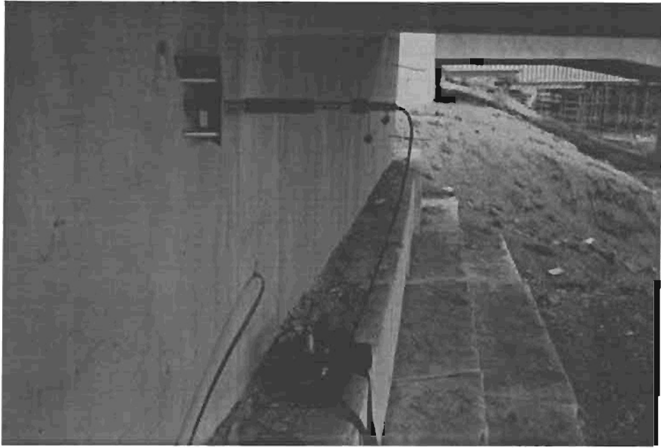
Photo 6: An Extensometer Electrical Sensor Head Installed at an Abutment Wall
