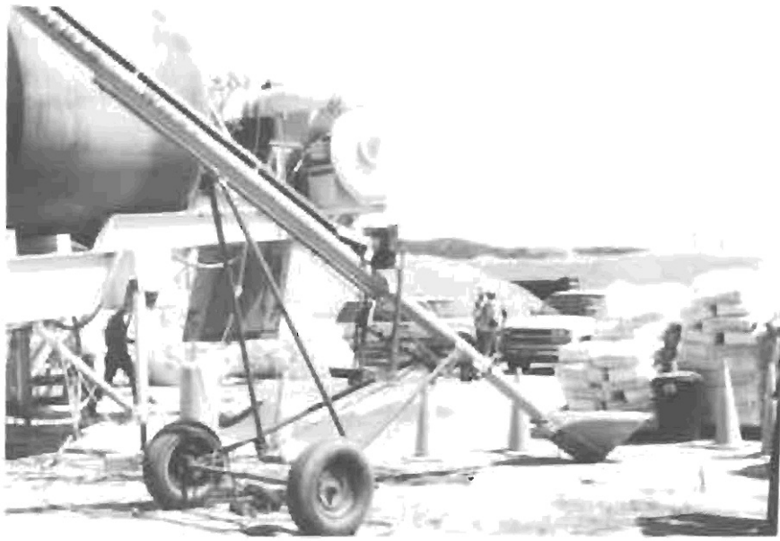
Figure 8. Auger System Initially Used for Vestoplast S.
